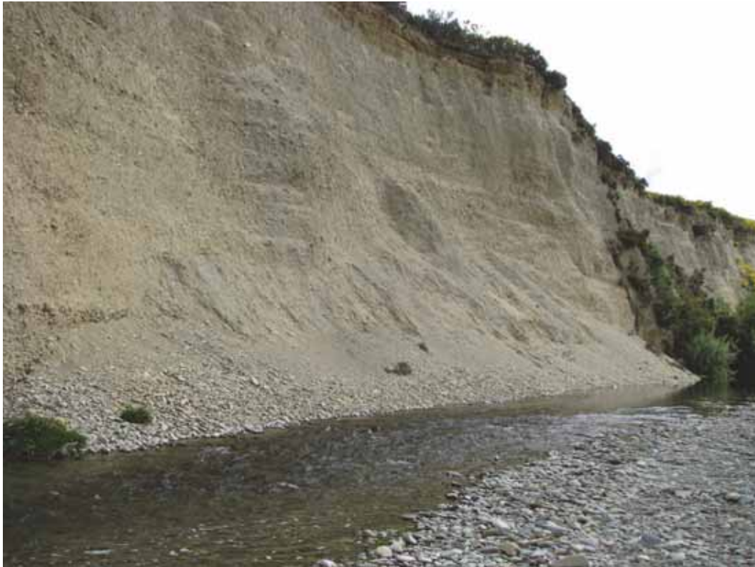
Figure 9. Area of active bank erosion on the South Branch of the Waianakarua River (between cross-section WA7S and WA8S), looking upstream, October 2013
