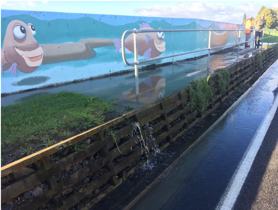
Figure 1 The College Road floodwall at Edgecumbe at 0814hrs on 6 April 2017. Structural failure of the floodwall occurred at approximately 0830hrs (photo credit: Tony Dunlop, Bay of Plenty Regional Council).
