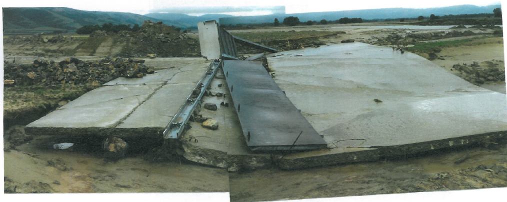
Figure 5 Some of the remnants of ORC's Riverside Spillway following failure of the collapsible section in December 1993
