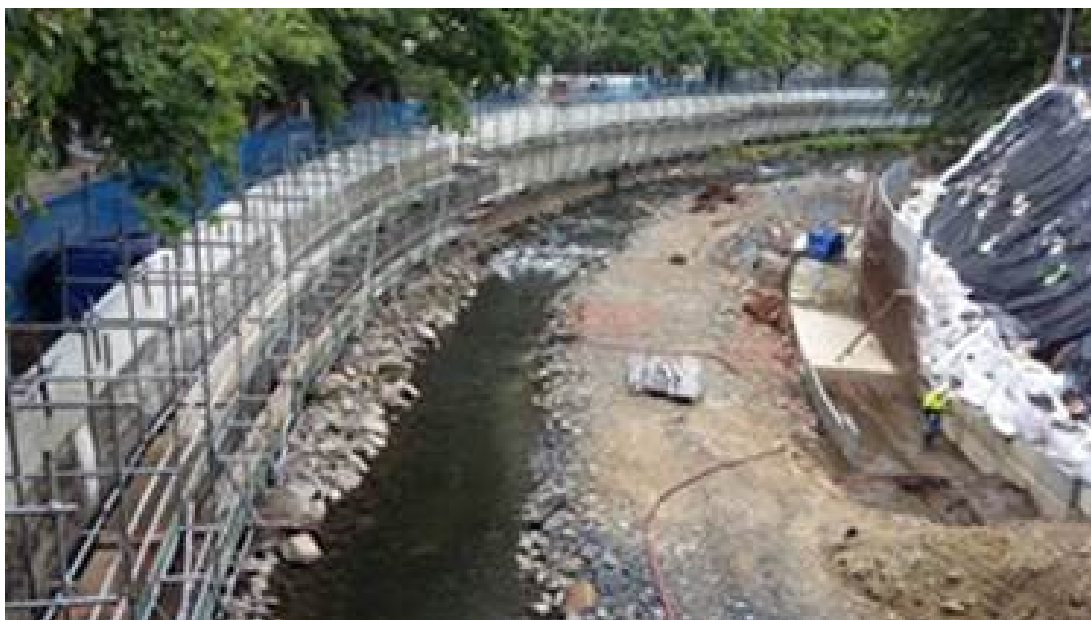
Figure 3: Leith Flood Protection Scheme works between Union Street and Leith Footbridge on 13 November 2017. The photograph is looking upstream.
