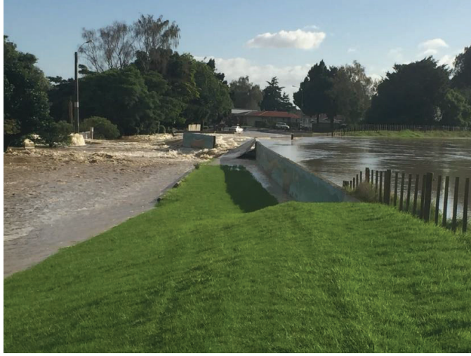
Figure 20: The breached Floodwall at Edgumbe, looking downstream; image file date-stamped 08:35 6 April, some 5 minutes after the breach (Source: Bay of Plenty Regional Council Contractor, 2017)
