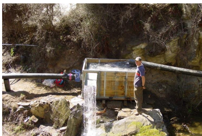
Figure 29: Waiwera Creek Intake
