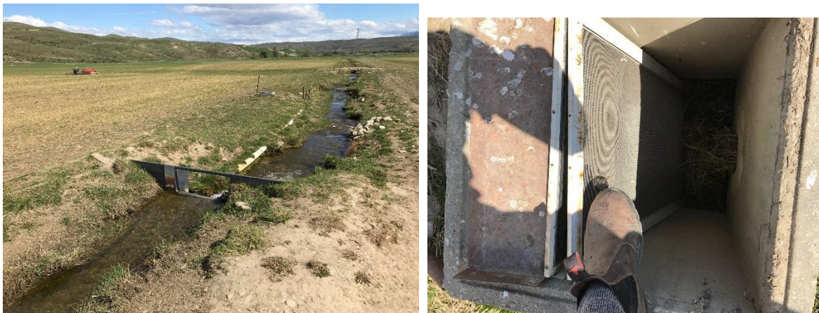
Coal Creek. Race diversion site and screen on intake
