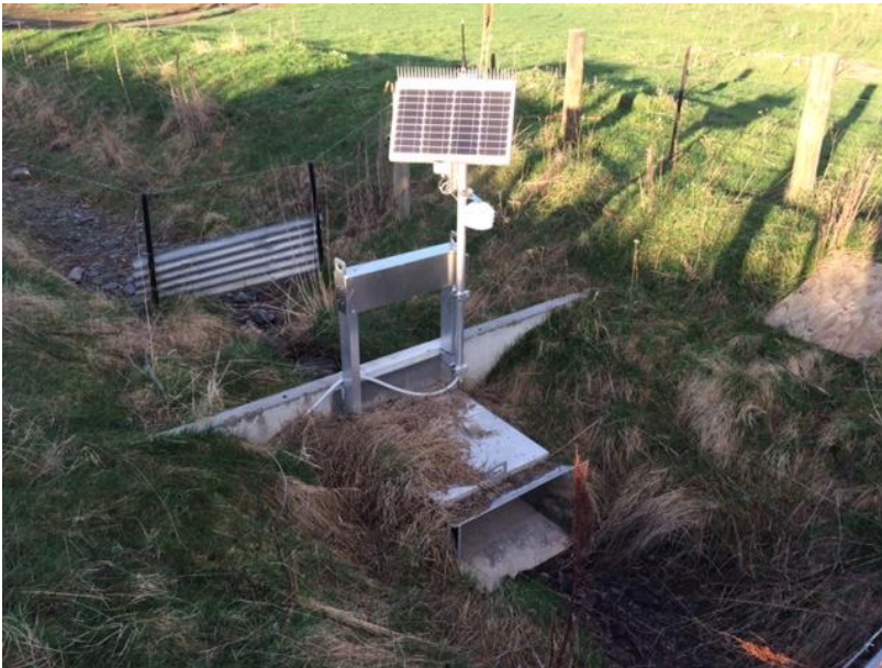
Combined measuring for Take Point 3 and 4
