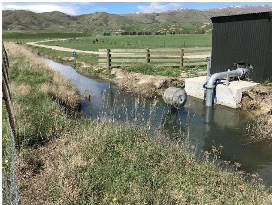
Screens on pumped intakes from Lindis race
