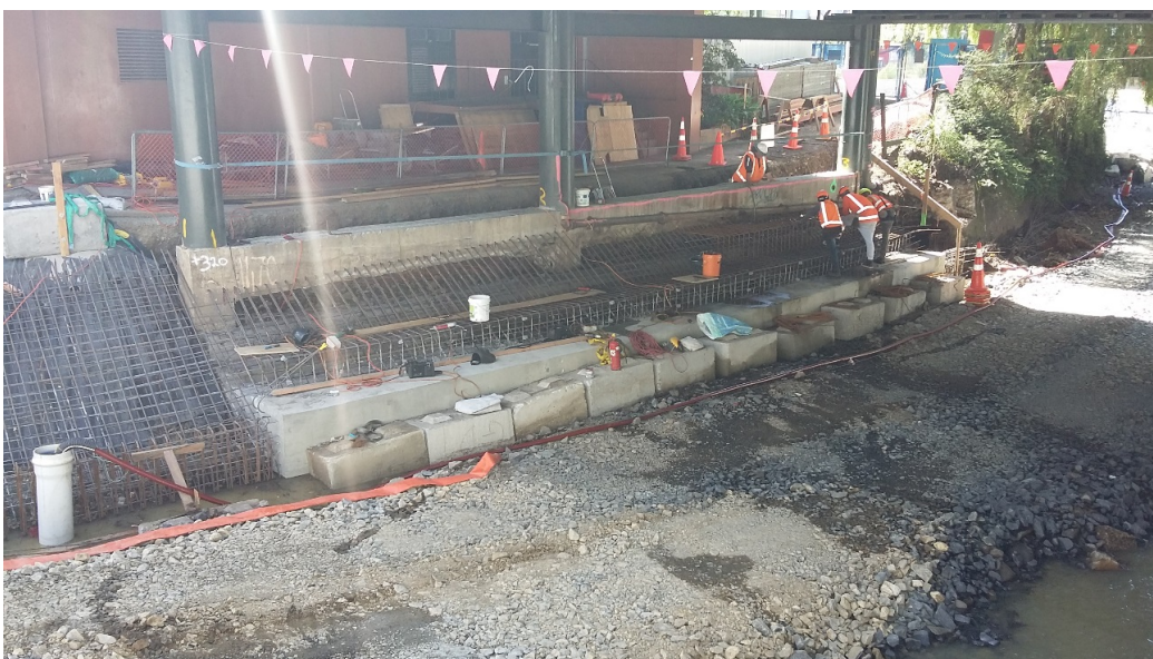
Figure 9: Leith Flood Protection Scheme works between Union Street and Leith Footbridge; this photograph was taken during low flows.
