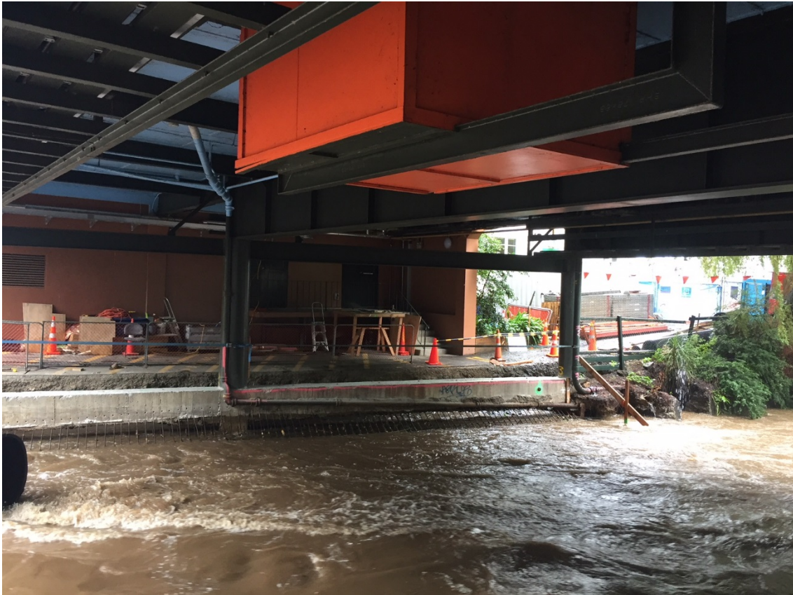
Figure 10: Leith Flood Protection Scheme works between Union Street and Leith Footbridge. The photographs in Figures 9 and 10 are looking towards the left bank below the ITS building. This photograph was taken on 1 February 2018 at a flow of approximately 48\text{m}^3/\text{s} ; peak flow during this event was 61\text{m}^3/\text{s} . The Scheme design flow is 171\text{m}^3/\text{s} .
