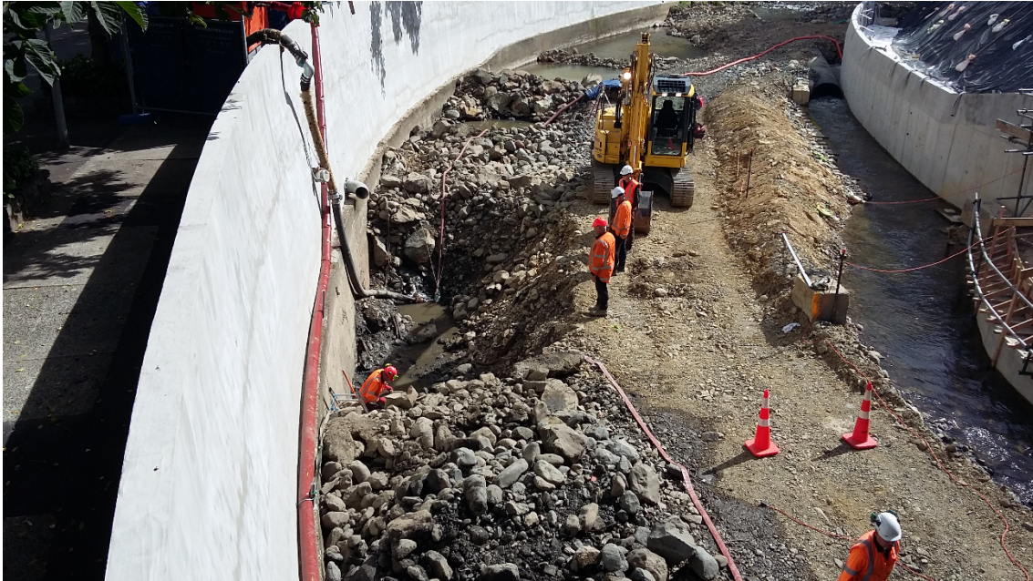
Figure 8: Works to foundation of Water of Leith right bank wall upstream of ITS building (13 March 2018). The photograph is looking upstream.
