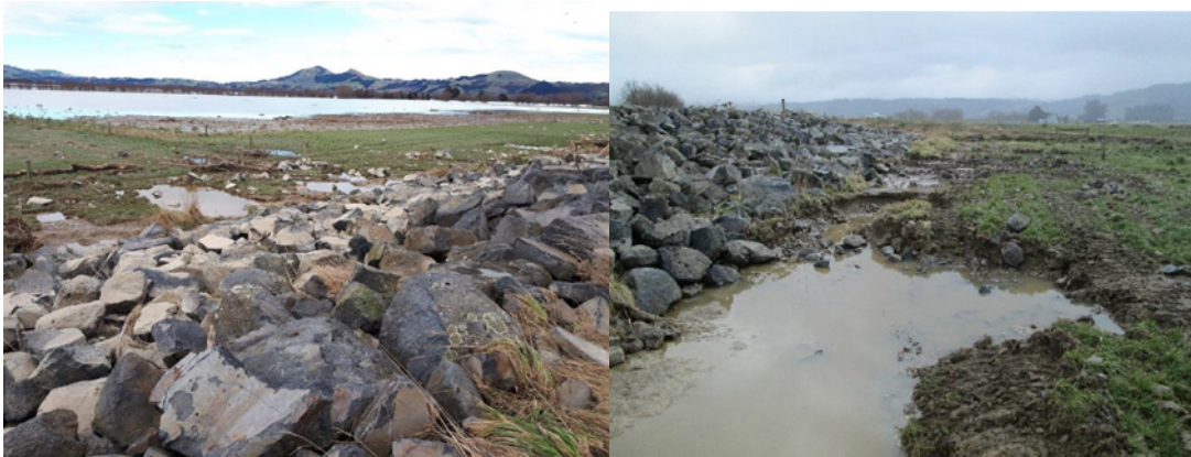
Figure 8 – Riverside Road Spillway showing scour damage post July 2017 flood.
