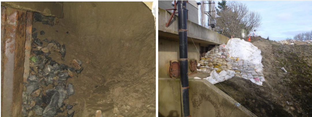
Figure 7 – Mill Creek Pump Station. Left Photo: Cavity scoured away within floodbank post July 2017 event. Right Photo: Sandbags installed during event to arrest seepage of floodwater through Taieri left bank floodbank.
