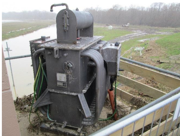
Photo 11: Silver Stream pumping station transformer.
