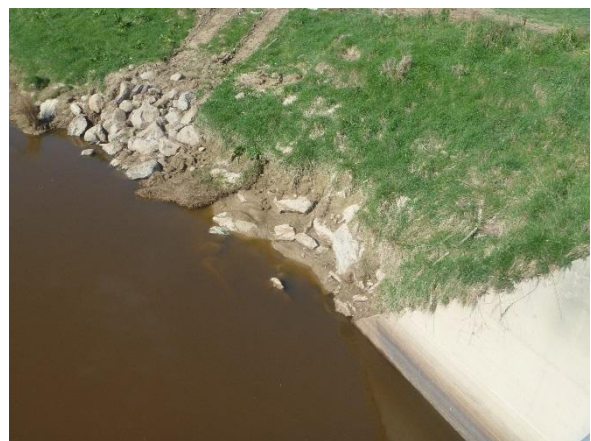
Photo 46: Recent scour and recent placement of rip rap rock.
