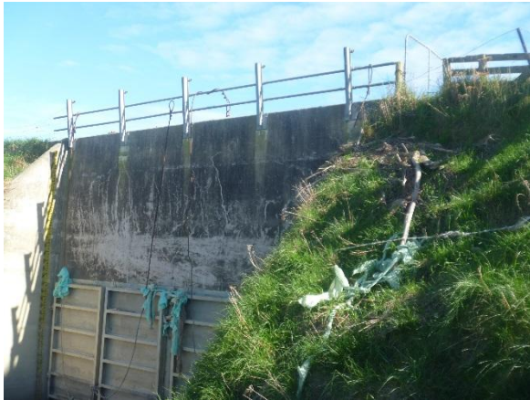
Photo 44: View of structure from the downstream. Missing hand rail and flood debris on gate visible.
