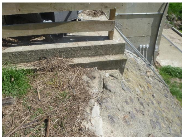
Photo 10: Displaced ground below the transformer slab previously repaired by concrete below the original slab in the vicinity of the recent seepage.
