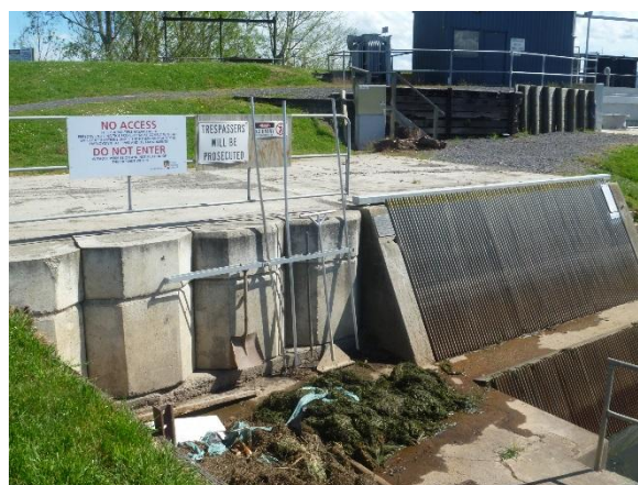
Photo 20: Pump intake area assessable to the public.
