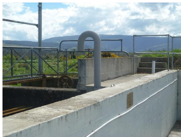
Photo 18: Low spot in crest wall approximately 600 mm high associated with pumping station reconfiguration work.
