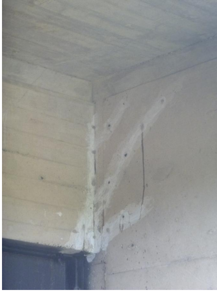
Photo 15: Flood gate bridge cracking – previously repaired.
