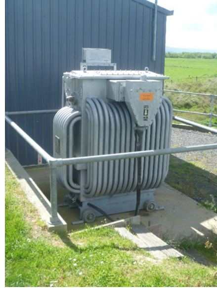
Photo 22: Waipori Pumping Station transformer.
