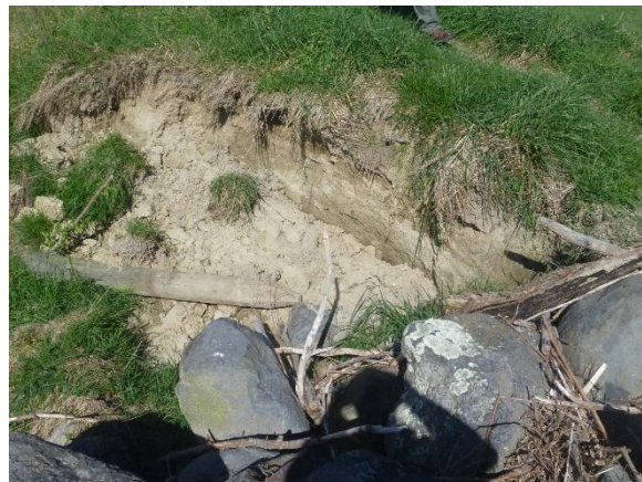
Photo 41: Right abutment damage from the July 2017 flood event. Location at significant risk of further damage.
