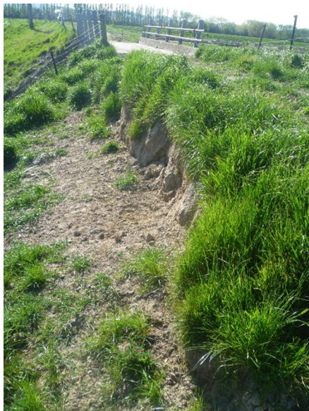
Photo 47: Damage to floodbank earth fill adjacent to the structure right hand side abutment.
