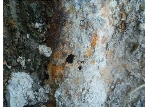
Photo 54: Corrosion at the invert of the Lower Pond Outlet invert near the inlet headwall. Indications are that a void is present behind the rust hole in the steel culvert and repair is warranted.
