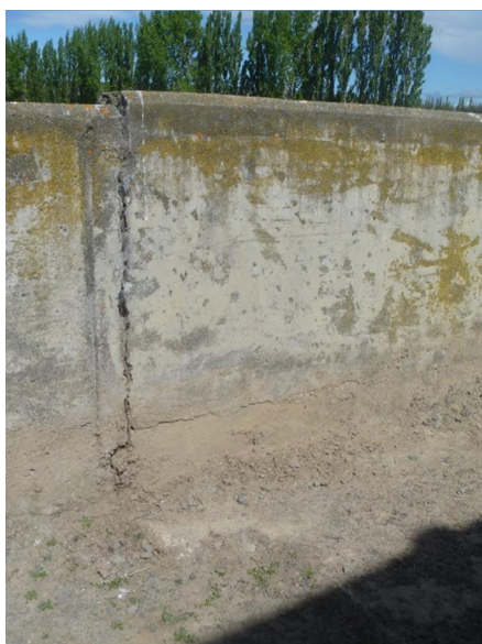
Photo 14: Cracking in parapet wall. Note inferred extent of original extent of concrete wheel stop at underside of parapet wall visible to the right of the right of the vertical crack.
