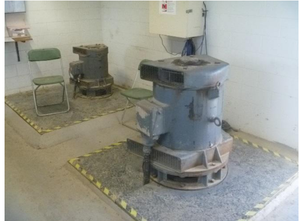
Photo 6: Pump motor – ORC report that the water level exceeded the floor level by about 0.2 – 0.3 m during the July 2017 flood event.
