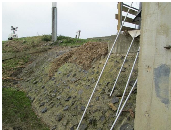
Photo 4: Cracking in grouted rock fill below the station transformer and location of historical seepage. Understanding is that seepage reported during July 2017 flood event emerged from top crack immediately below formed face of transformer foundation.
