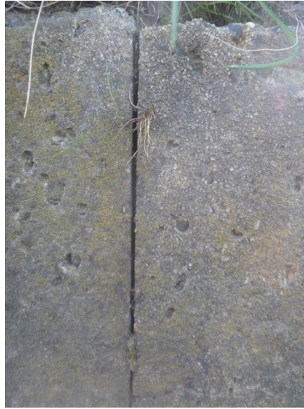
Photo 8: Construction joint in head wall at rising main outlet. Note apparent movement. Location of interest for tell-tale installation.
