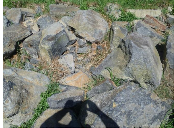
Photo 34: Damaged rip rap near the crest– note loss of rock.
