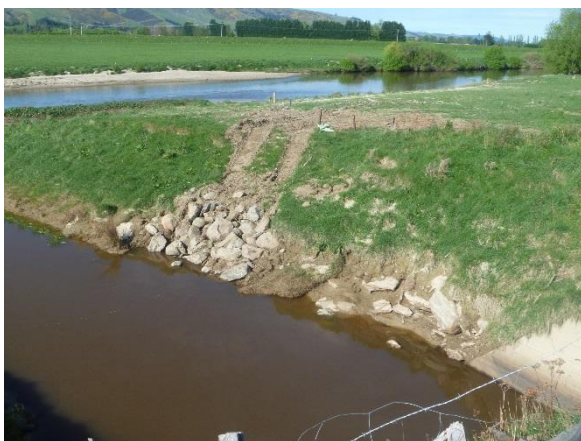
Photo 45: View towards Taieri River from A1 Outfall. Note recent scour and recent placement of rip rap rock.
