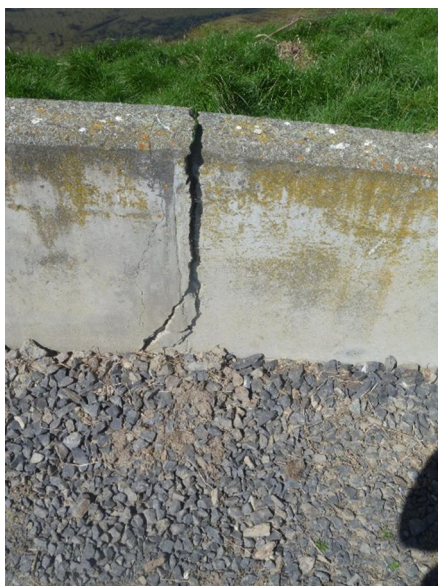
Photo 12: Parapet wall cracking from vehicle access. Installation and monitoring of tell-tale device recommended.
