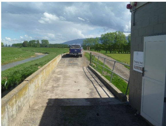
Photo 1: Looking downstream along Silver Stream towards River road (10 October 2017). Note cracking in parapet wall on left coincident with inferred extent of sheet pile support to underside of gravity gate and bridge structure.
