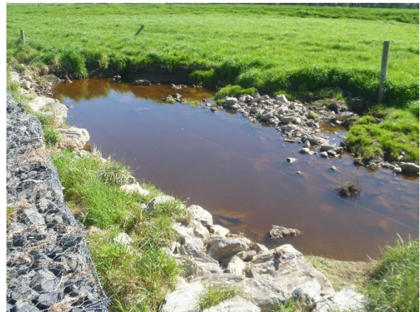
Photo 36: Scour damage downstream of spillway gated section.
