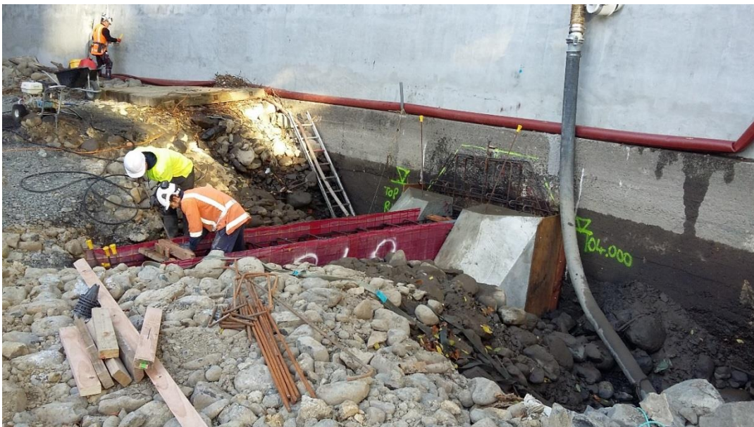
Figure 3: Installation of weir and buttresses within Water of Leith near the wall on the south side of the channel (the outside of the river bend).
