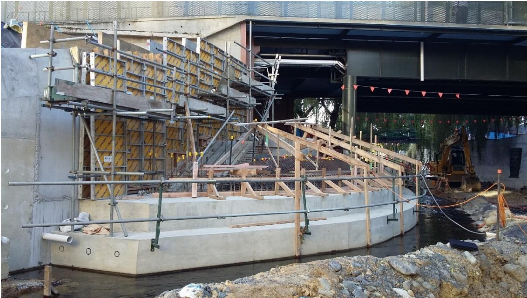
Figure 2: Construction of walls and terraces upstream of and beneath the Information Technology Services (ITS) building (north side of channel).
