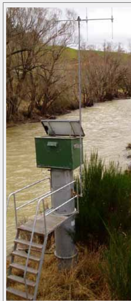
Flow monitoring station Taieri River at Tiroiti
