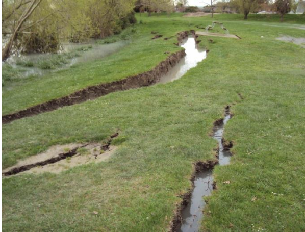
Figure 7.4 Lateral spreading on the true-left bank of the Kaiapoi River, after the Christchurch magnitude 6.3 earthquake.
