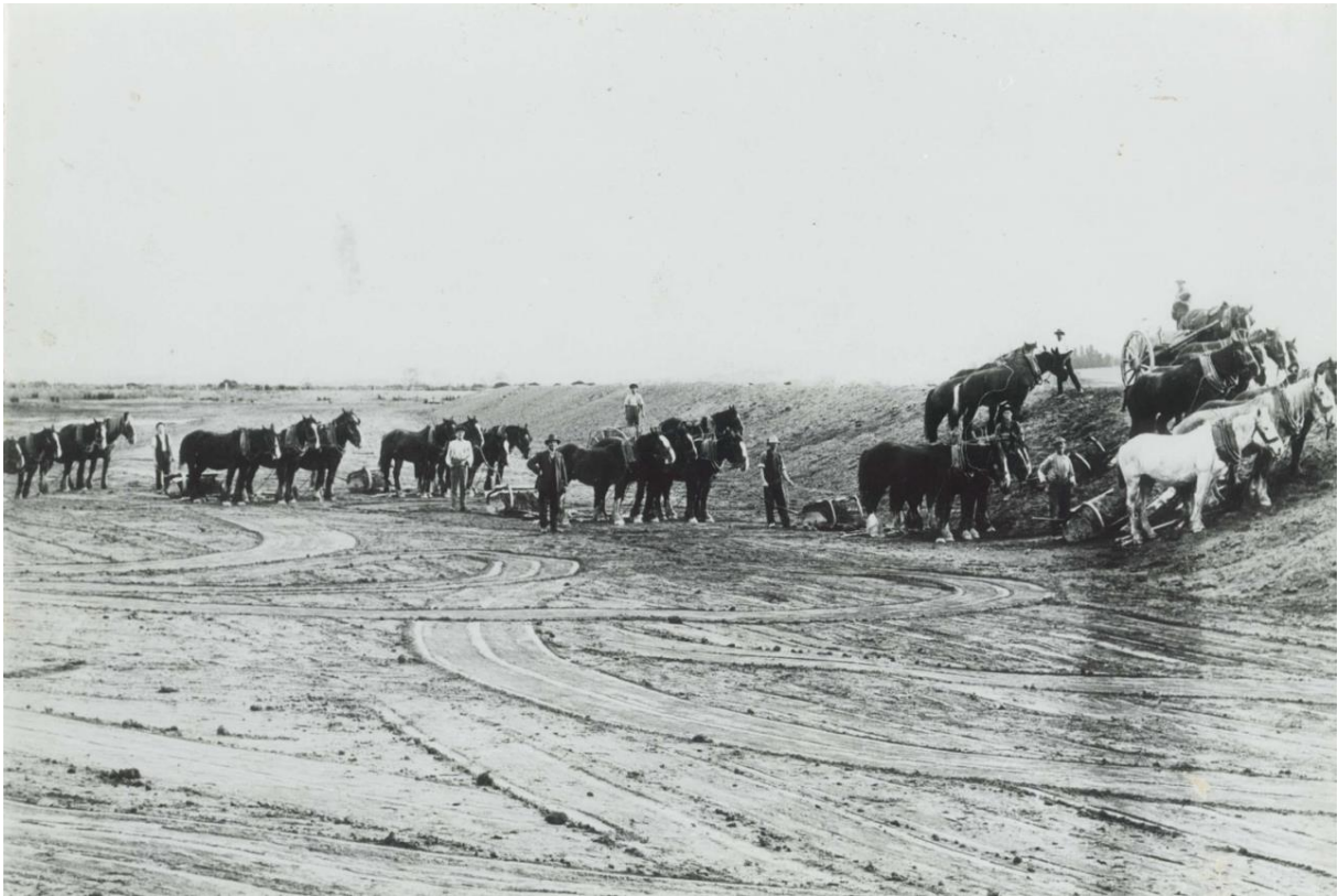
Figure 2.4 Early construction of the Contour Channel on the West Taieri Plain (circa 1915).
