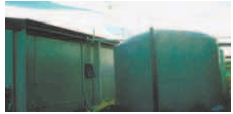
Storm water collection.
