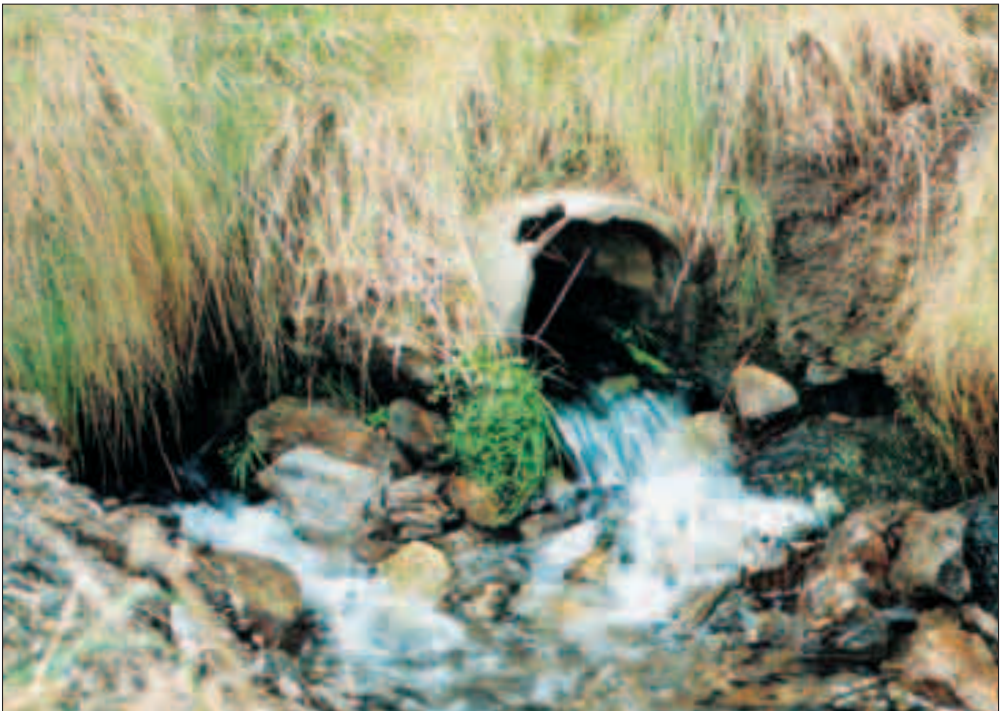
Culvert with rocks to create fish pass on Owhiro Stream, East Taieri
