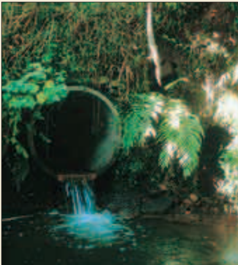
Poorly designed culvert (not level with bed, no fish access)
