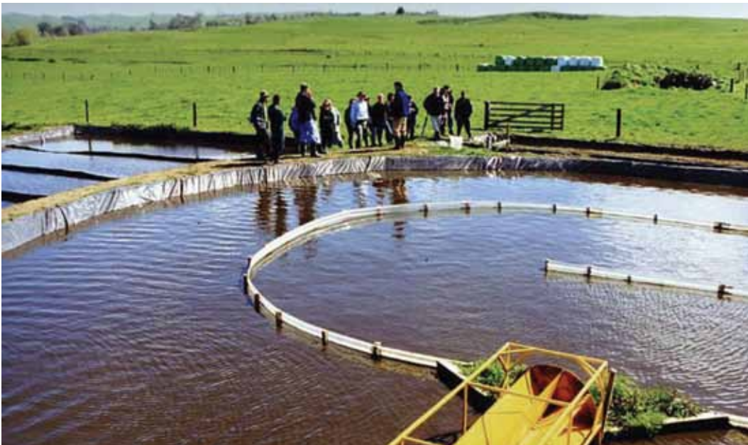
Figure 1 Advanced effluent pond system
