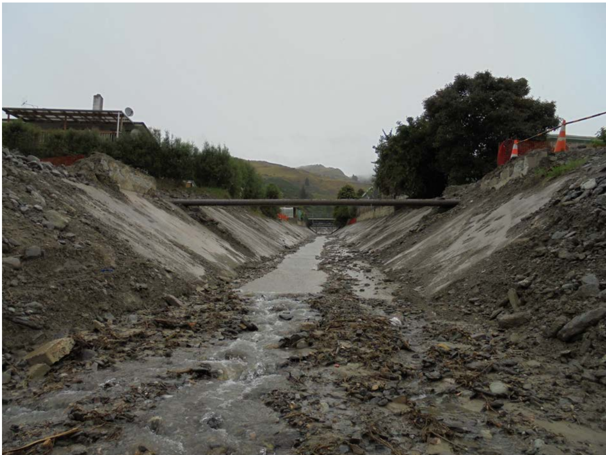
Figure 3.13 The cleared concrete debris flow channel two weeks after the debris flows of 26 th November 2017 (Photo: S.Dellow 13/12/2017).
