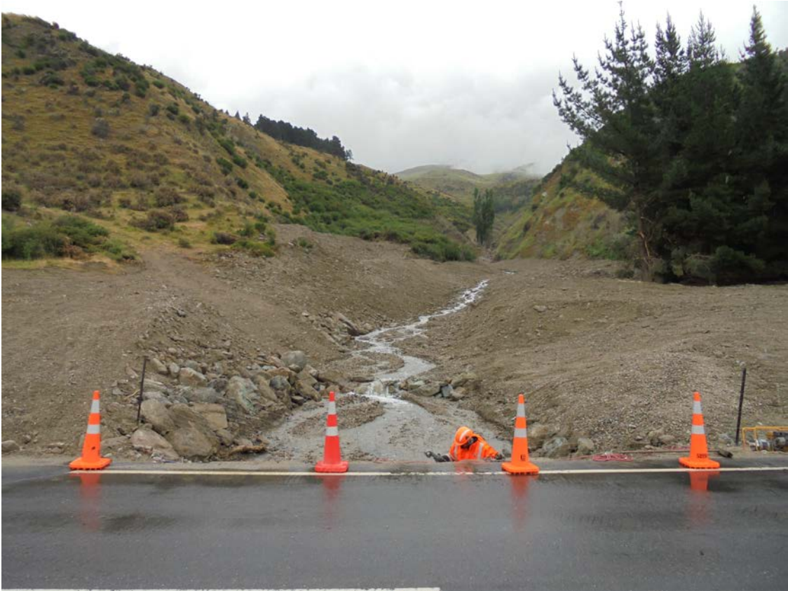
Figure 3.3 Black Jacks Creek looking upstream from the culvert over SH8. The height of the un-vegetated channel banks provides some indication of the amount of aggradation caused by the debris flows close to the fan-head (Photo: S.Dellow 13/12/2017).
