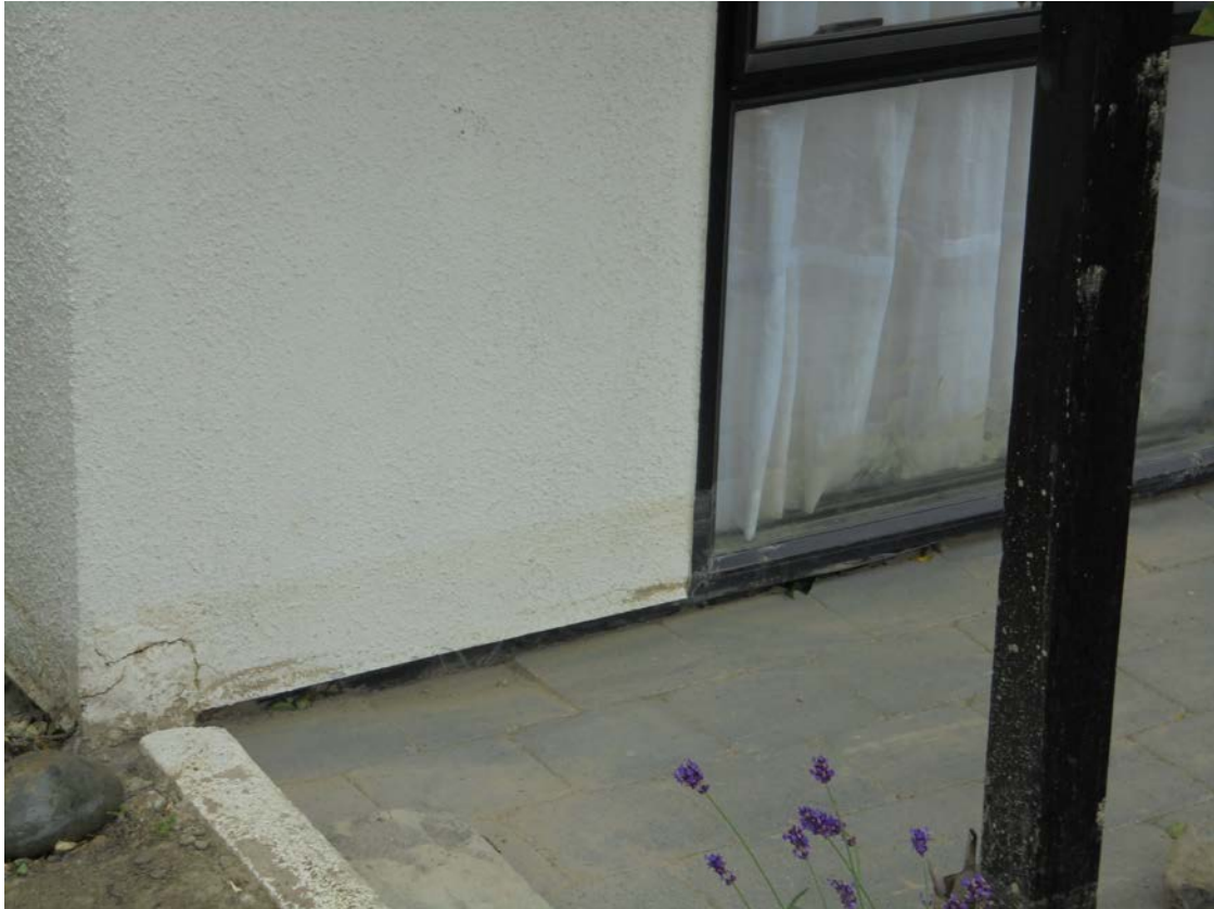
Figure 4.2 Evidence of silt and water damage on a building exterior. Depth of inundation appears to be about 100 mm (Photo: S.Dellow 13/12/2017).
