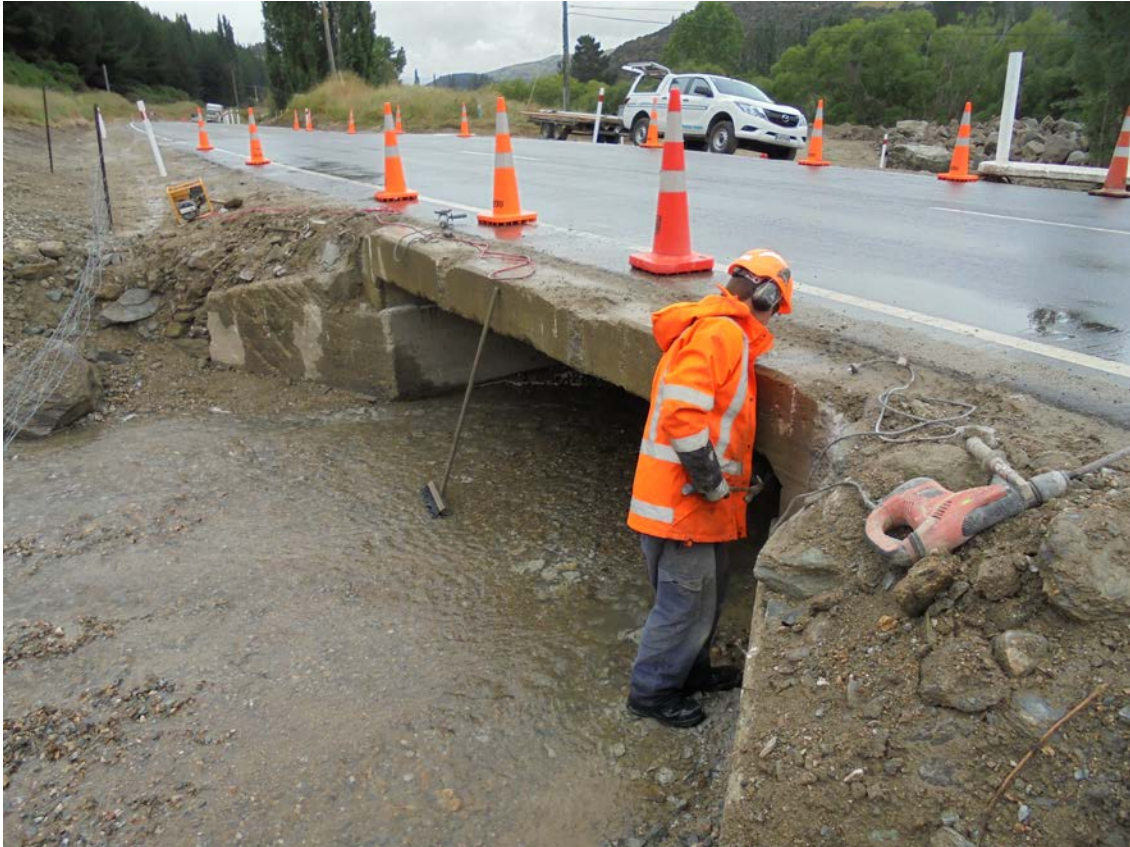
Figure 3.4 The culvert beneath SH8 at Black Jacks Creek. Note the height of the culvert in relation to the size of the largest boulders in the figure below (Photo: S.Dellow 13/12/2017).
