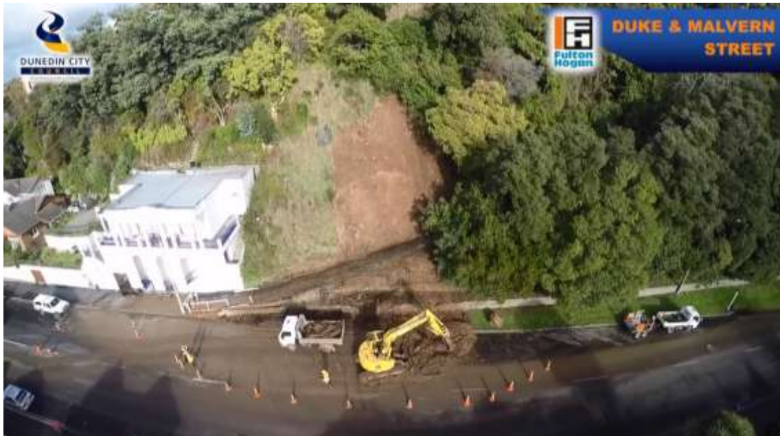
Figure 32 Aerial view showing a cleanup underway to remove landslide debris at the base of the Bullock Track and on Duke Street. Source: DCC/Fulton Hogan
