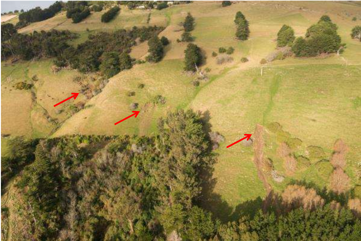
Figure 13 Aerial view of the slopes above the Howard Street slides on 16 June 2015. The approximate locations of the surficial slides shown in this photograph (red arrows) are shown in Figure 12.
