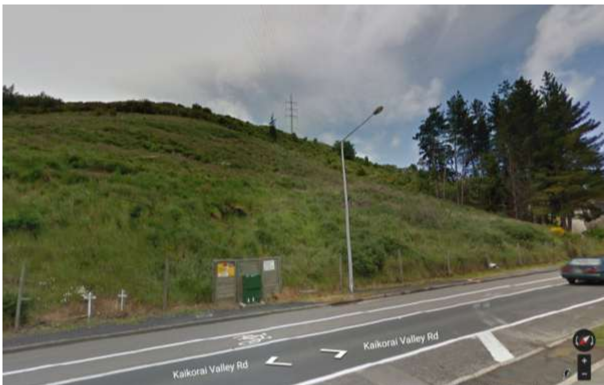
Figure 36 View of the 577 Kaikorai Valley Road landslide from Kaikorai Valley Road (Google Street View)
