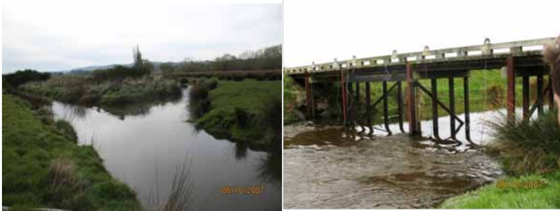
Figure 8 The left hand photo shows Stony Creek converging with the diversion channel and the right hand photo shows the Lake Tuakitoto outlet sill.
