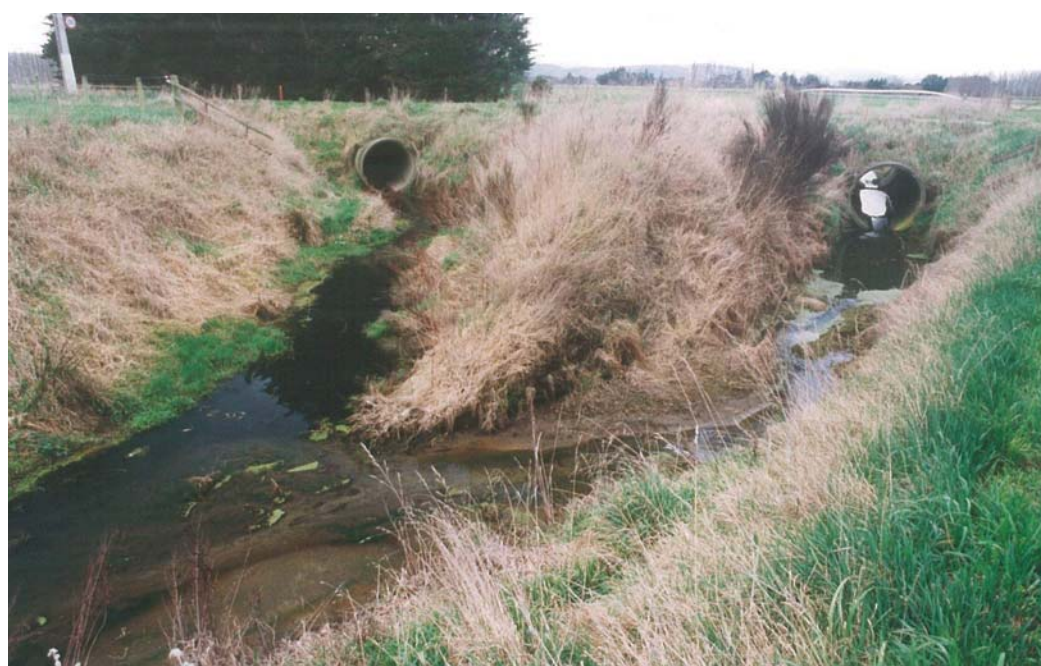
Figure 5.9 Black enriched water from the #28 Drain (left) entering the Main Drain at Miller Road
