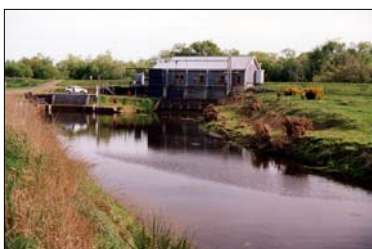
Site 21 Main Drain @ Waipori Pumping Station
