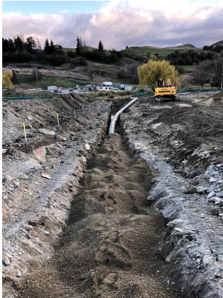
Figure 8. Installation of the pipe at Millbrook’s Dagleish Farm development to enable transfer of water from the Arrow Irrigation Company scheme to Mill Creek. View to the south.
