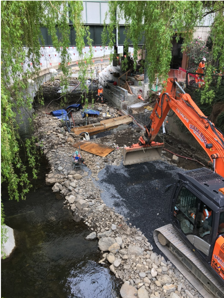
Figure 9. Looking downstream (top) and upstream (bottom) along the bed of the Water of Leith near the Information Technology Services (ITS) Building (9 October 2018). The river is temporarily diverted adjacent to the right-bank wall.
