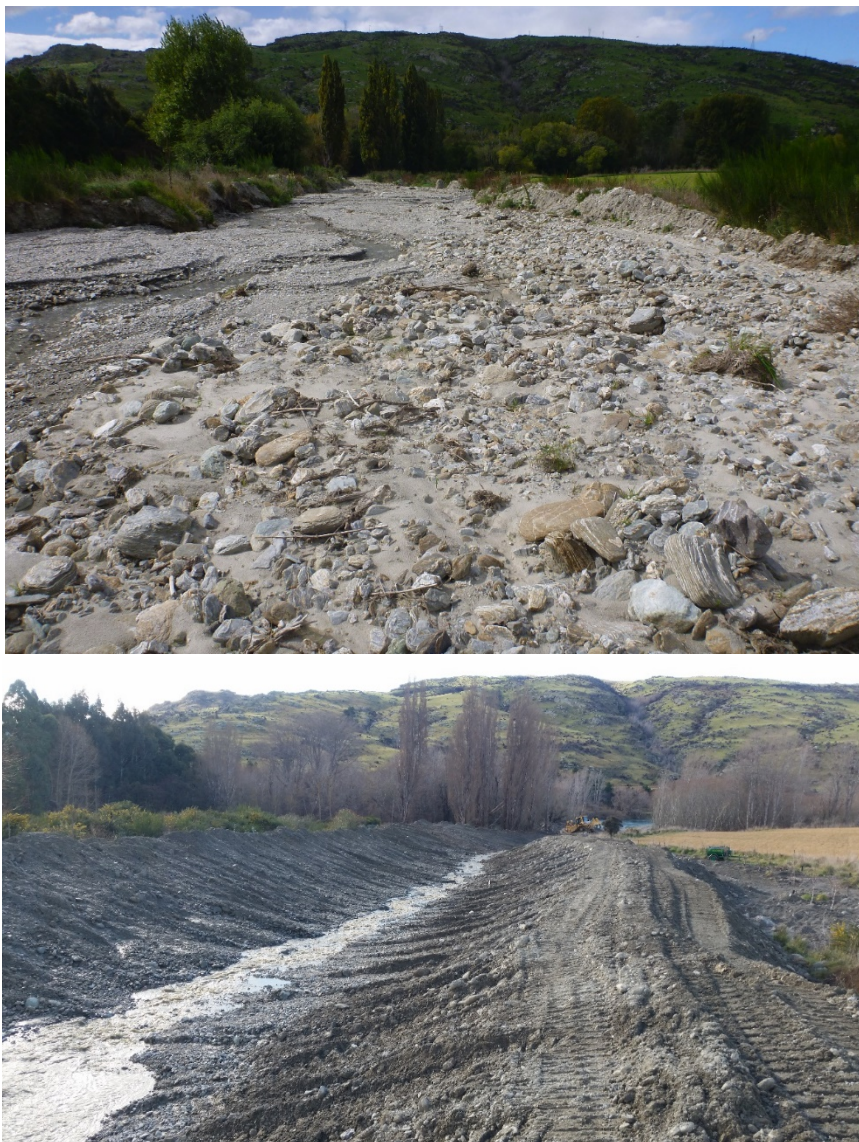
Figure 3. View down the lower reach of Stephensons Creek (south of Roxburgh) before (top) and after (bottom) channel restoration works undertaken by ORC.
