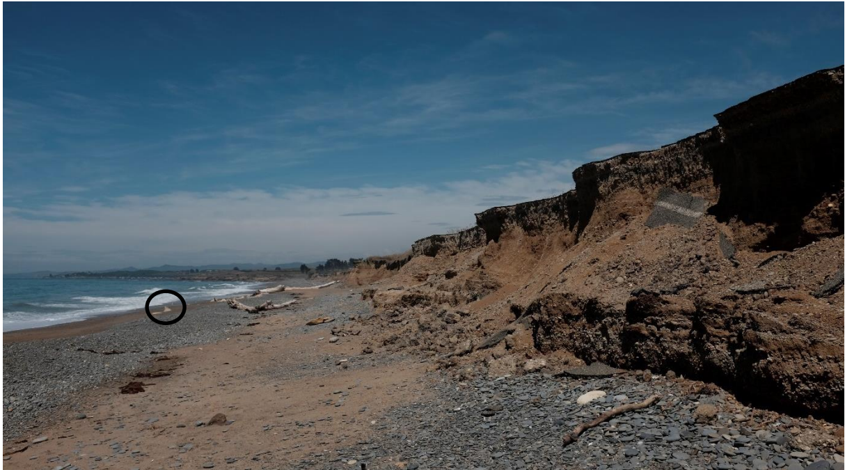
Figure 3-12: Example of unconsolidated cliff morphology: Beach Road. Note remnants of the old coastal road on the cliff top and scattered light-coloured blocks from a failed rip-rap wall in the distance (circled).
