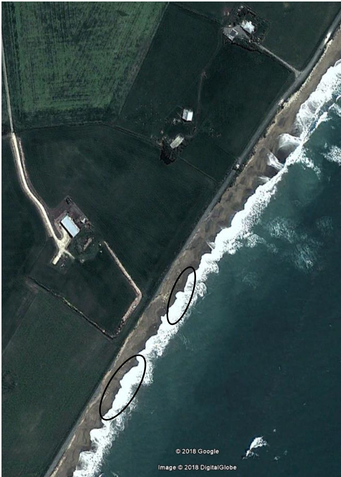
Figure 4-2: Riprap section on Beach Road viewed on satellite imagery of 03/10/2012. The view is the same as shown on Figure 4-1. Note the material of the failed riprap scattered on the foreshore (circled in black). Imagery source: DigitalGlobe.
