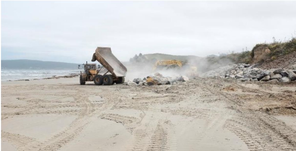
Figure 3-1: Armouring of the backshore cliff on Katiki Road (7/12/2017).
