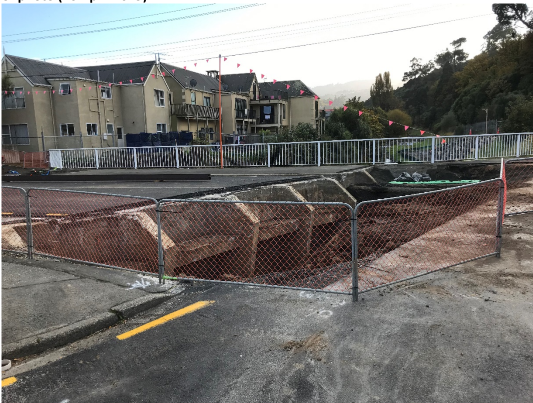
Figure 5: Excavation of ground behind eastern (true left) abutment of Dundas Street Bridge (26 April 2019)
