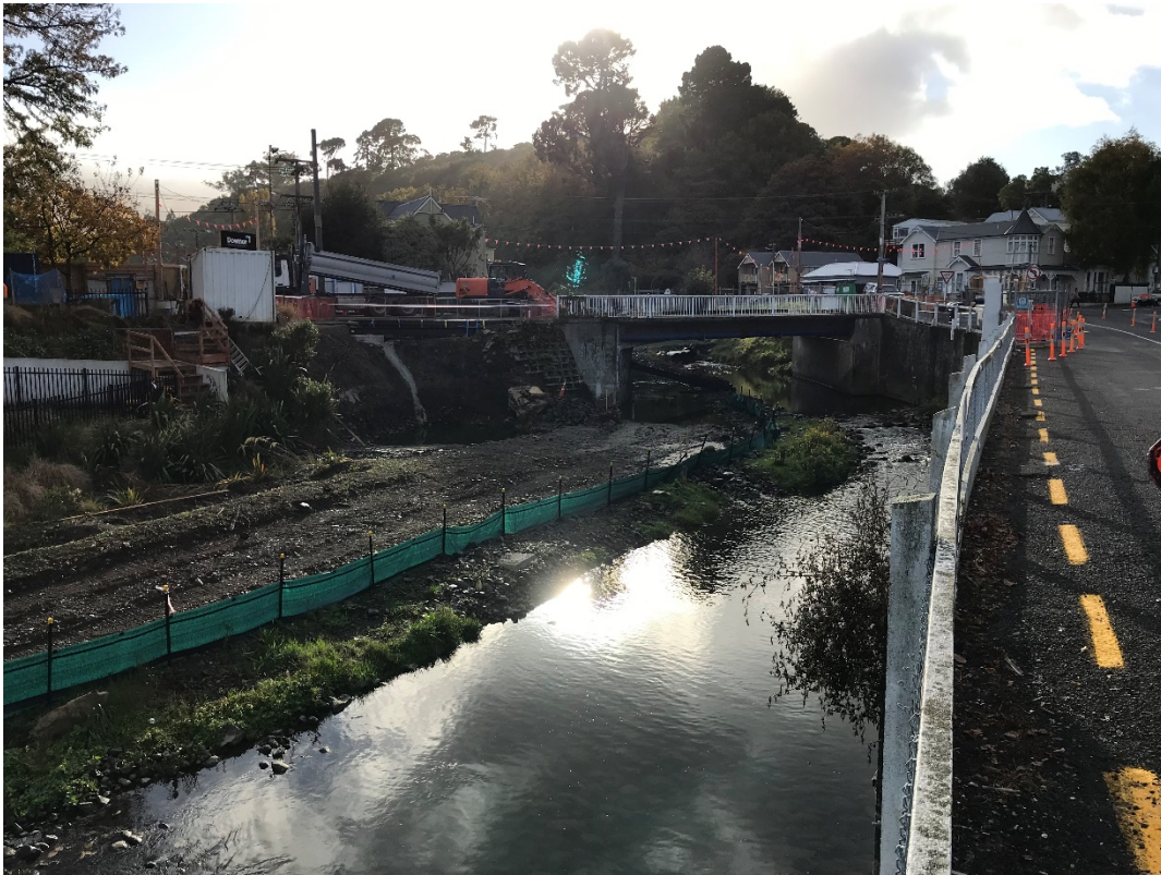
Figure 4: Dundas Street Bridge. Excavation of western (true right) abutment underway at left of photo (26 April 2019)
