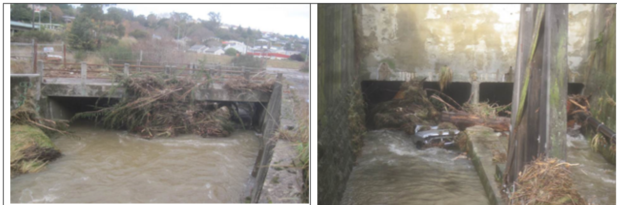
Figure 4: Example of channel blockage in June 2015 flood event – Left: Tree and debris trapped under the bridge at Burnside. Right: Car and tree lodged in culvert beneath SH1 at Burnside.
