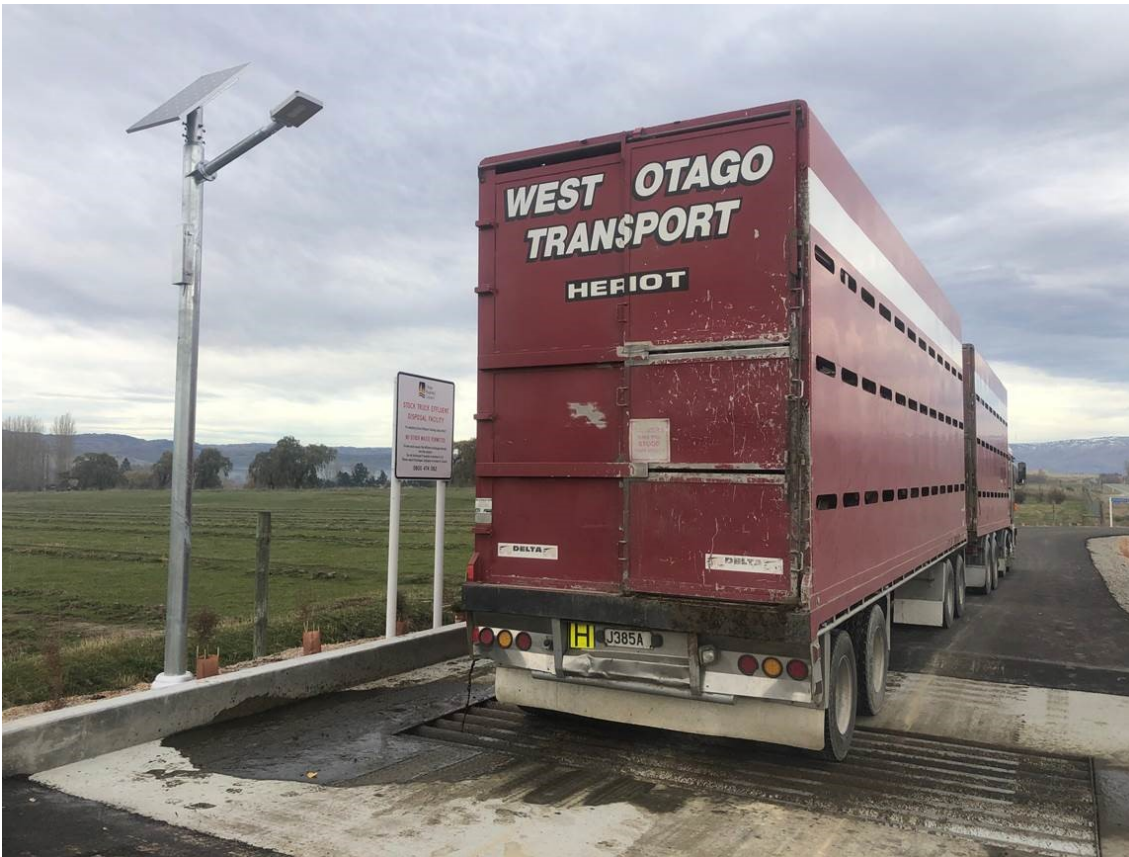
Figure 11: Stock truck discharging effluent into the SH85 (Brassknocker Road) STED on 26 May 2019 (photograph courtesy Bruce Robertson, Road Transport Logistics Ltd, Tapanui)
