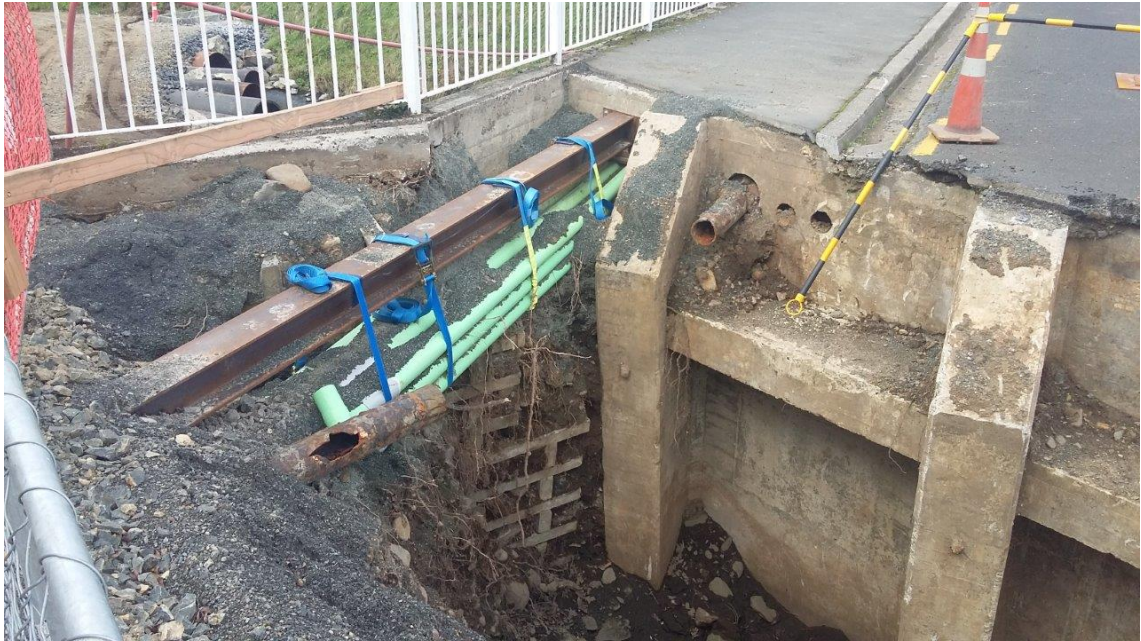
Figure 8 Excavation and communication ducts (green pipes) at western (right) abutment of Dundas Street Bridge.
