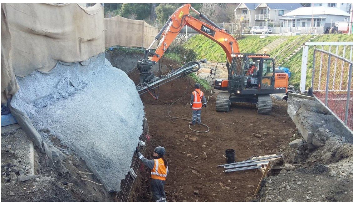
Figure 6 Ground pinning and Shotcrete ground stabilisation on western side of Water of Leith (looking upstream, bridge at right).
