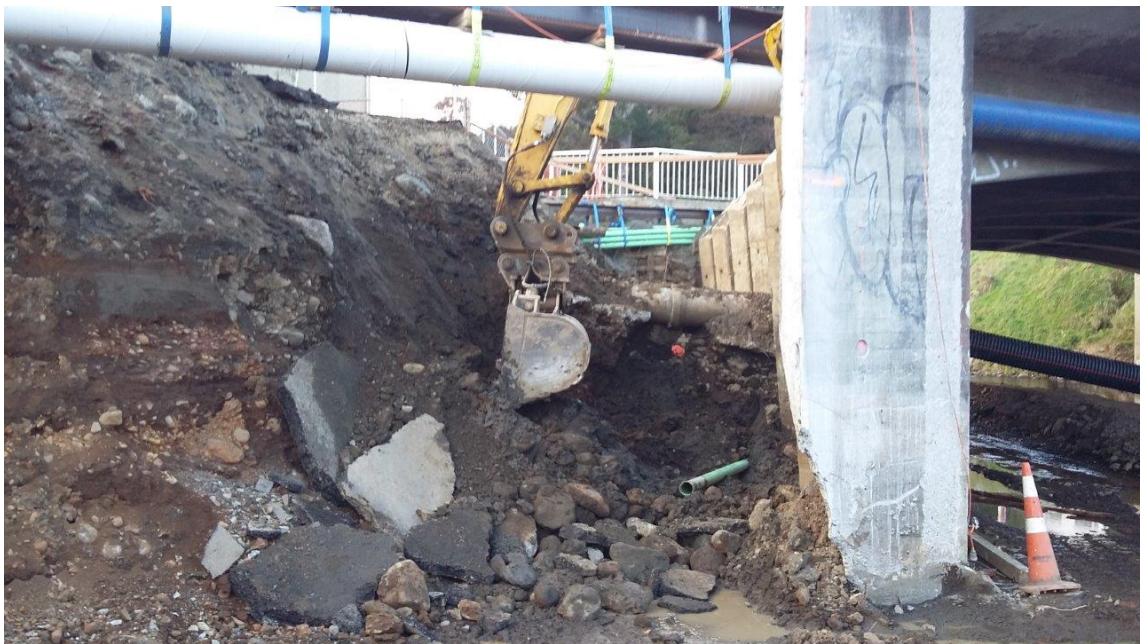
Figure 5 Looking upstream to excavation behind western (right) abutment of Dundas Street Bridge.
