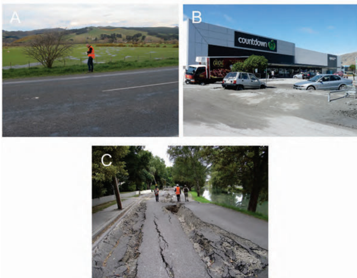
Figure 2.1 Photos illustrating some effects of liquefaction and lateral spreading. A: Relatively minor liquefaction effects in a paddock near Taitapu, with pods of grey sand/silt that issued from the ground during the 2010 Darfield Earthquake. GNS Science VML ID: 1398421; D.J.A. Barrell, 5 th Sept 2010. B: Severe liquefaction effects at Ferrymead, eastern Christchurch, where vast amounts of sand/silt issued from the ground, causing localised subsidence, during the 2011 Christchurch Earthquake. EQC/GNS Science VML ID:164424; A. King, 24 th Feb 2011. C: Lateral spreading and ground subsidence along a river bank in Avonside, eastern Christchurch, resulting from the 2011 Christchurch Earthquake. EQC/GNS Science VML ID: 149293; R.D. Beetham, 4 th March 2011.
