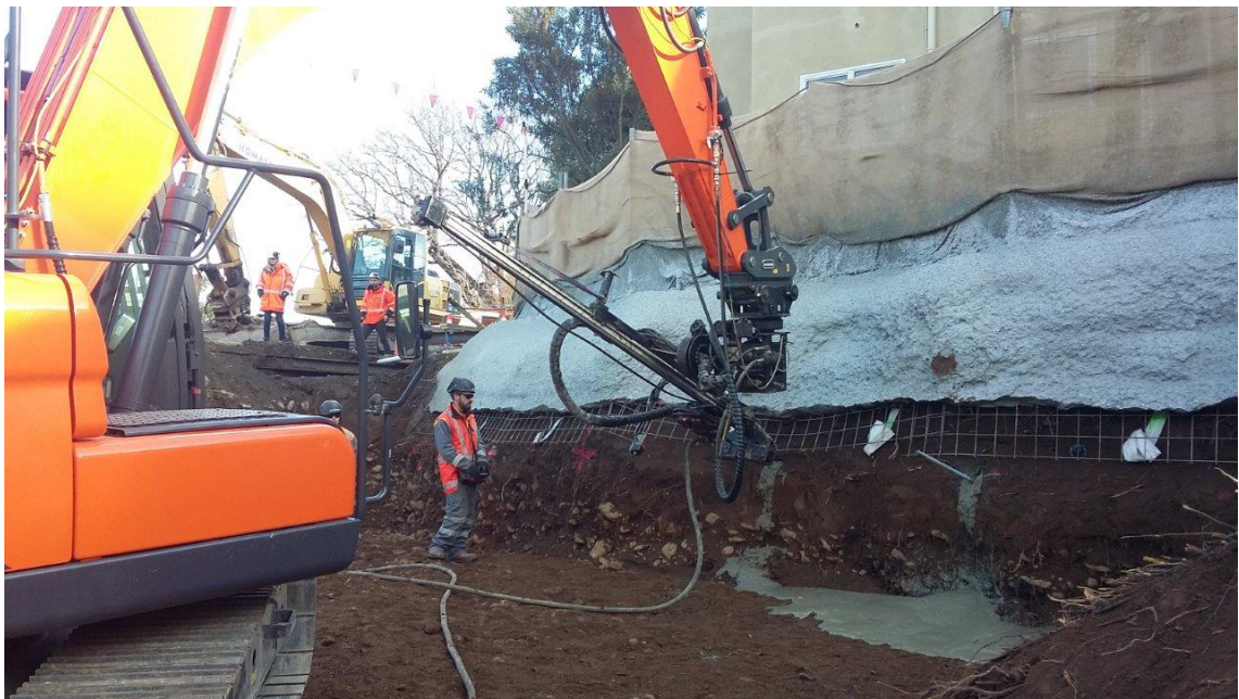
Figure 7 Ground pinning and Shotcrete retaining works on western side of Water of Leith, upstream of Dundas Street Bridge. The top of the Shotcrete is at the level of the pre-existing river bed (prior to channel widening).
