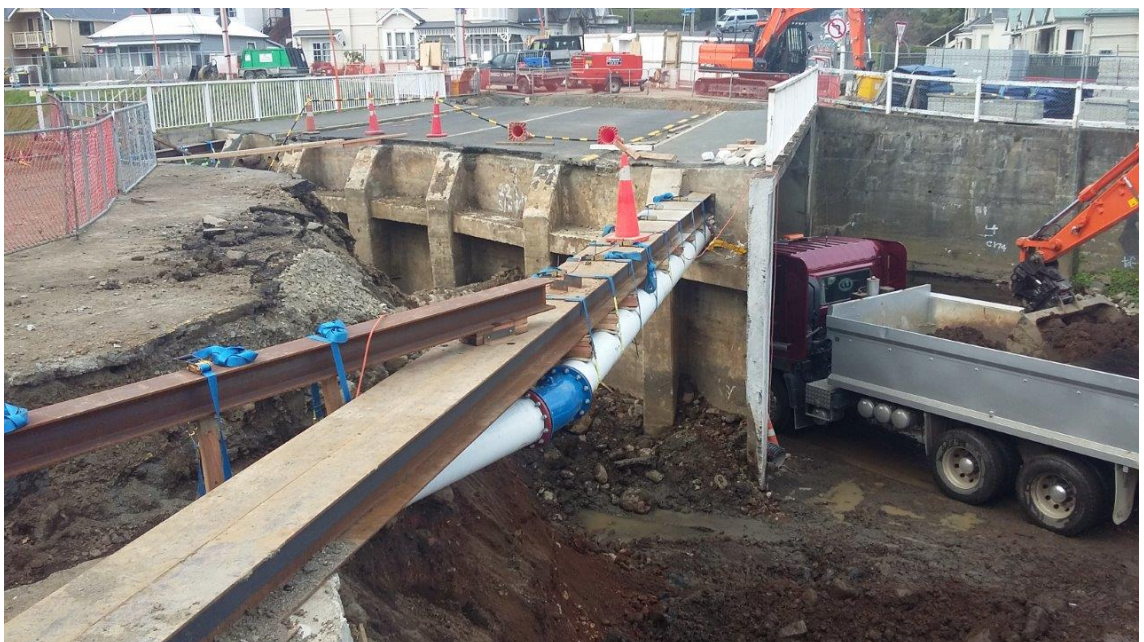
Figure 3 Western (right) abutment of Dundas Street Bridge, Dunedin. Dunedin City Council water main (white pipeline) and temporary steel support beam in foreground.
