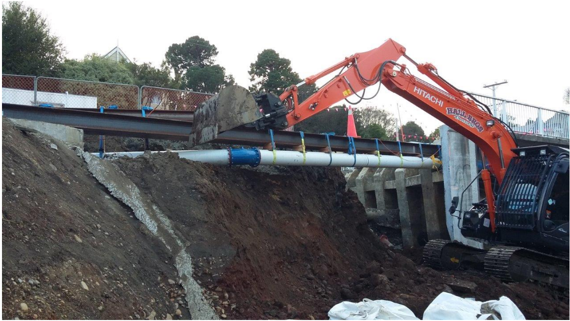
Figure 4 Looking upstream at western (right) abutment of Dundas Street Bridge, Dunedin. Dunedin City Council water main (white pipeline) and temporary steel support beam in foreground.
