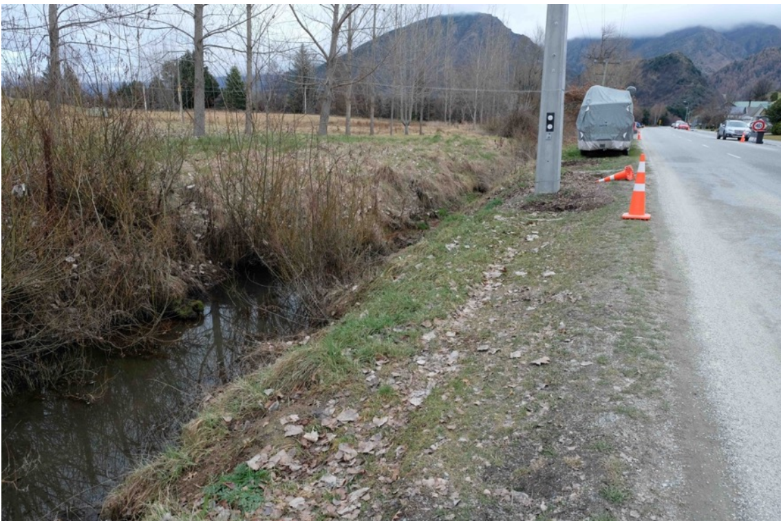
Figure 40 Roadside ditch beside McDonnell Road, Arrow Town near Pump station 19.
