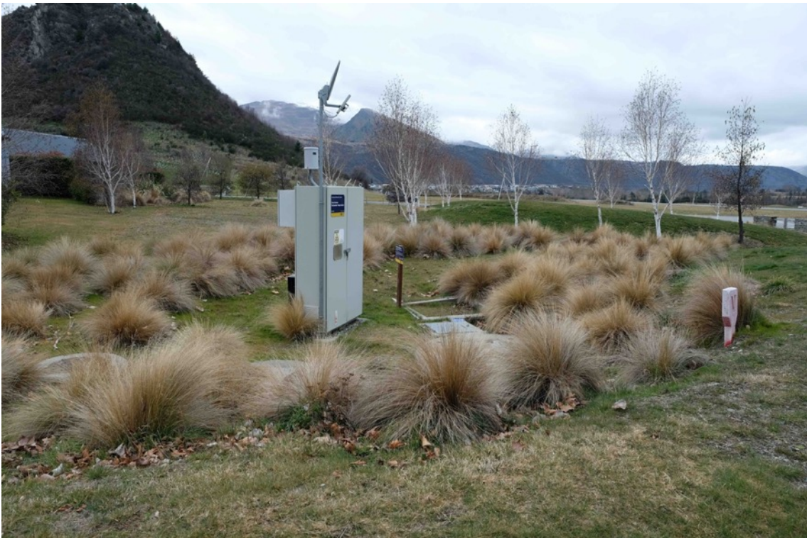
Figure 42 Pump station 20 beside Essex Avenue, Arrow Town.
