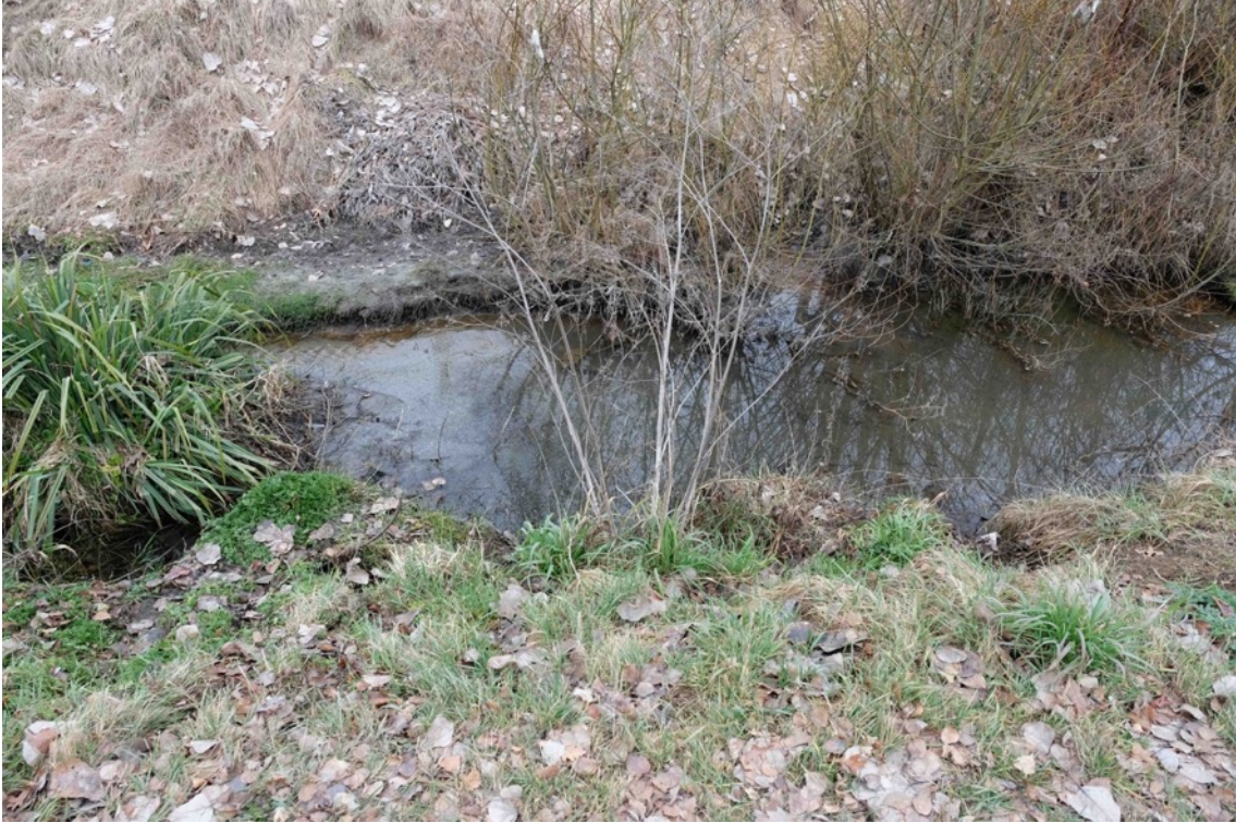
Figure 41 Roadside ditch beside McDonnell Road, Arrow Town near Pump station 19.
