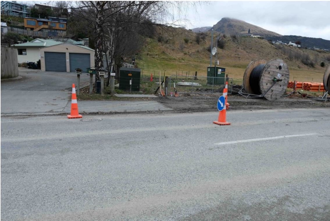
Figure 39 Pump station 19 beside McDonnell Road, Arrow Town.
