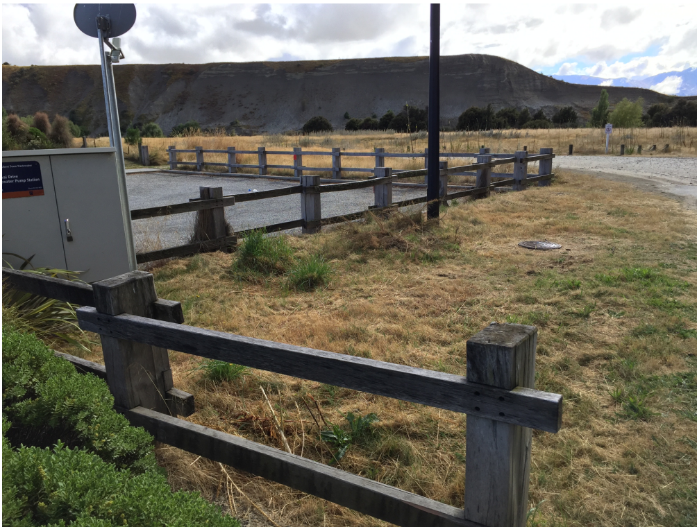
Figure 28 Pump station 11 on Gunn Road, Albert Town.
