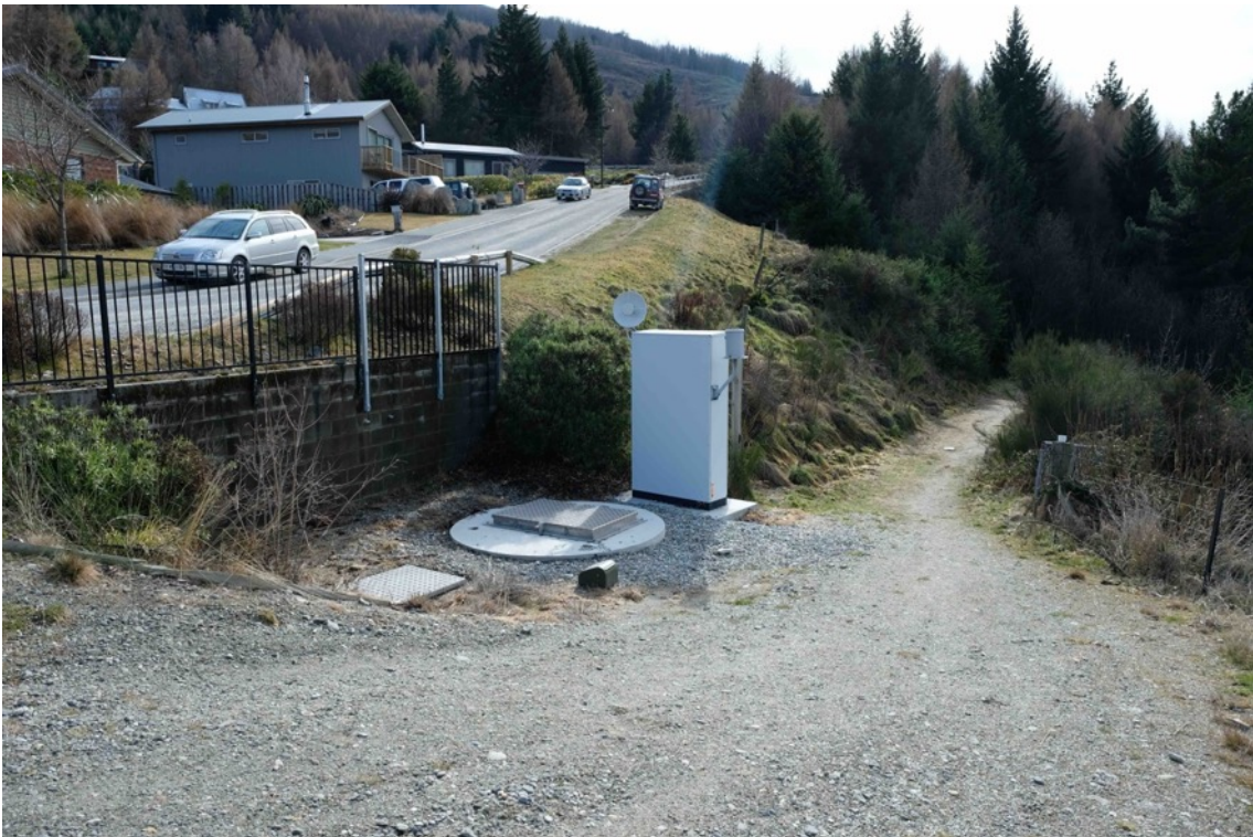
Figure 44 Pump station 21 beside Atley Road, Arthurs Point near the Shotover River.
