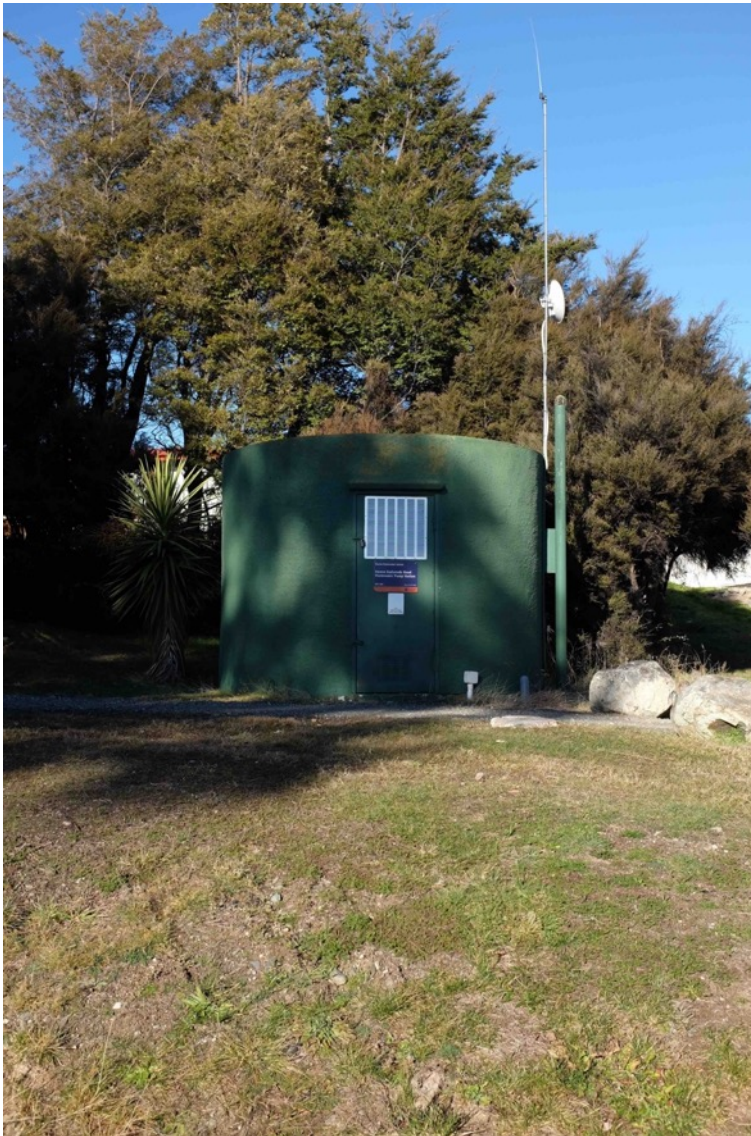
Figure 60 Pump Station 32 on Hāwea esplanade track on the shore of Lake Hāwea.
