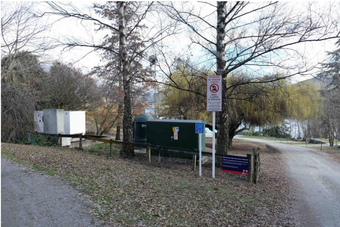
Figure 58 Pump Station 31 with Lake Hayes in the background.
