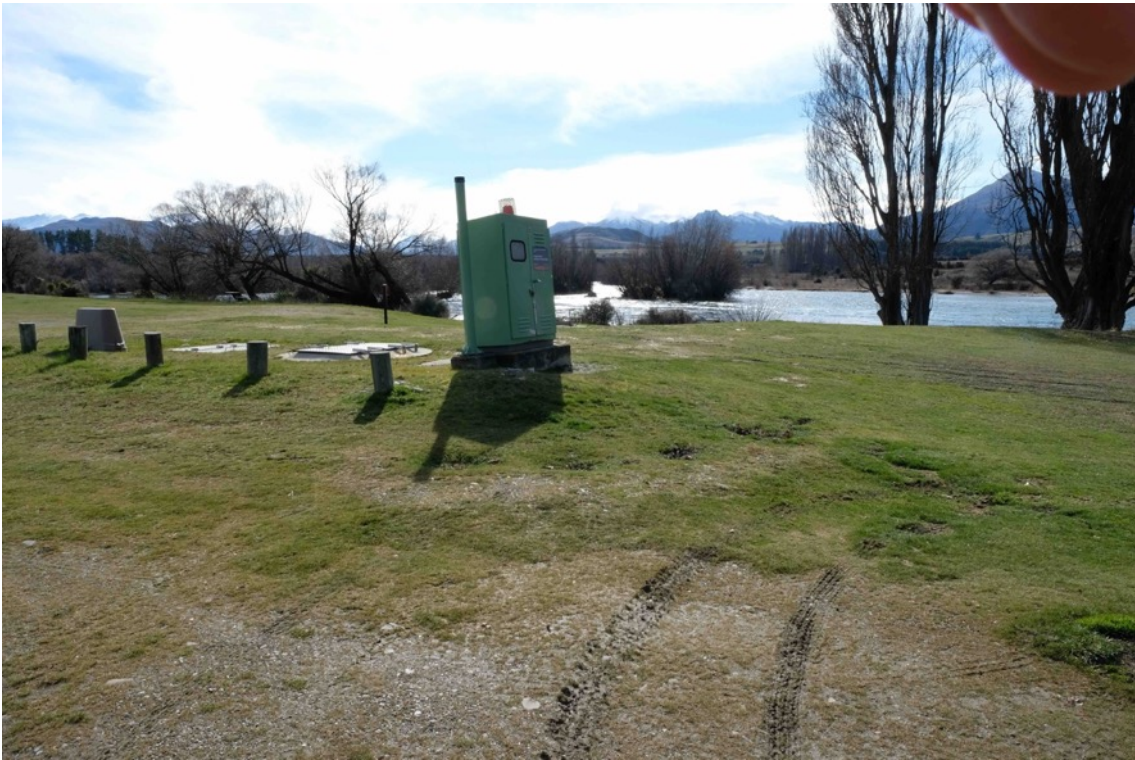
Figure 26 Pump station 10 on Wicklow Terrace (Albert Town) with Clutha River in background.
