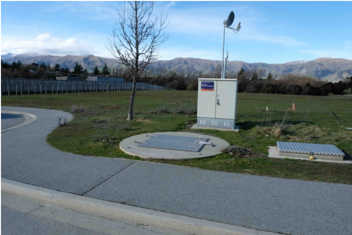
Figure 32 Pump station 16 on Harris Place, Luggate.
