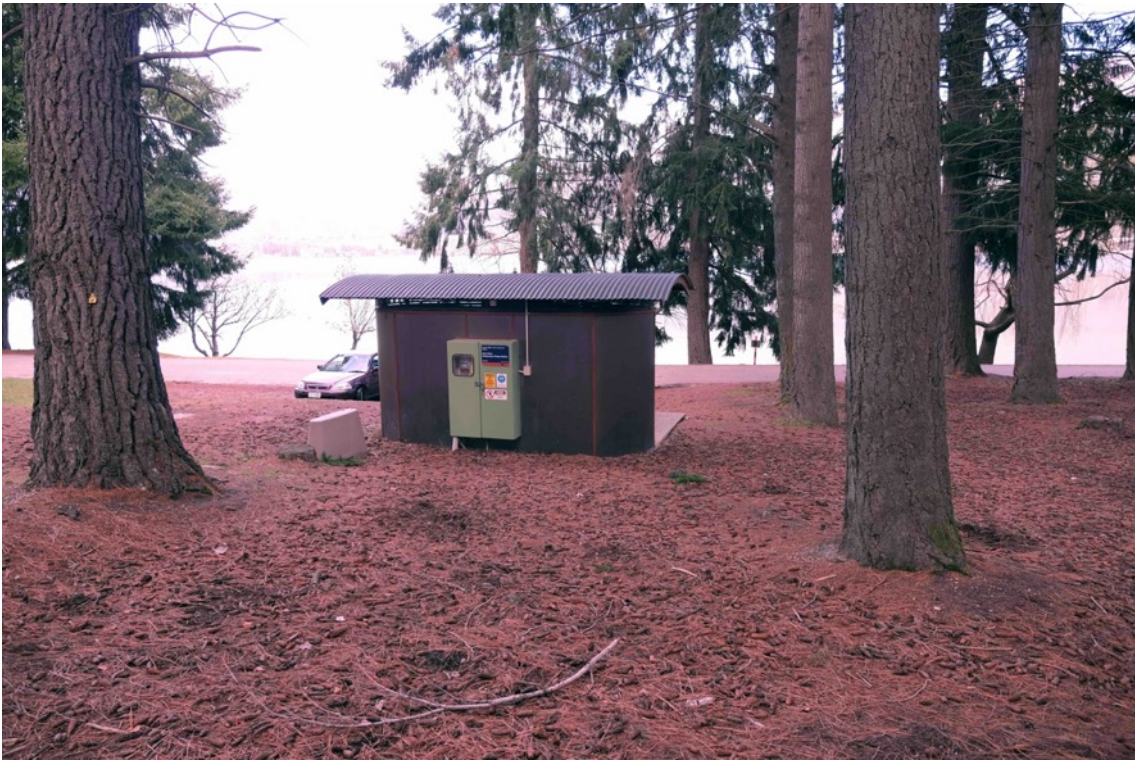
Figure 20 Pump station 3 located at Eely Point with Lake Wanaka in background.
