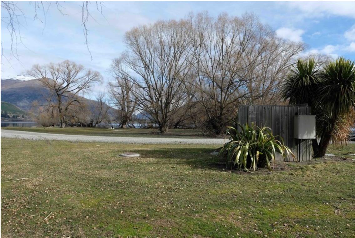
Figure 56 Pump Station 30 (foreground) looking towards Lake Hayes.
