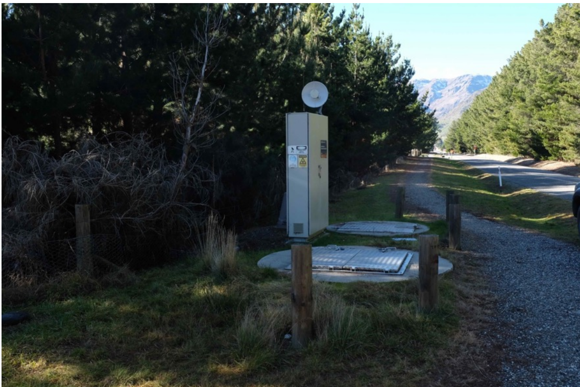
Figure 65 Pump Station 35 on Cemetery Road near Lake Hāwea.
