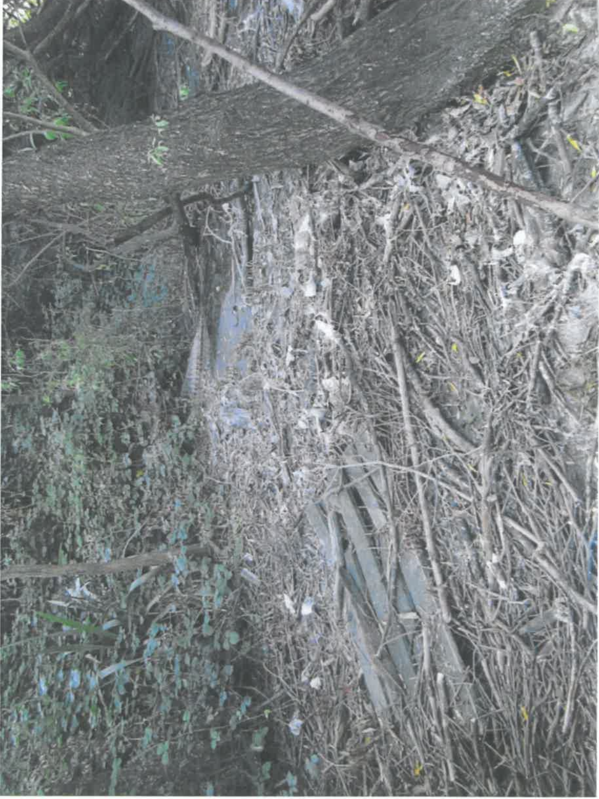
View of stormwater pipe outlet (centre of photograph) where the sewage discharge occurred. Note sewage debris in foreground.
