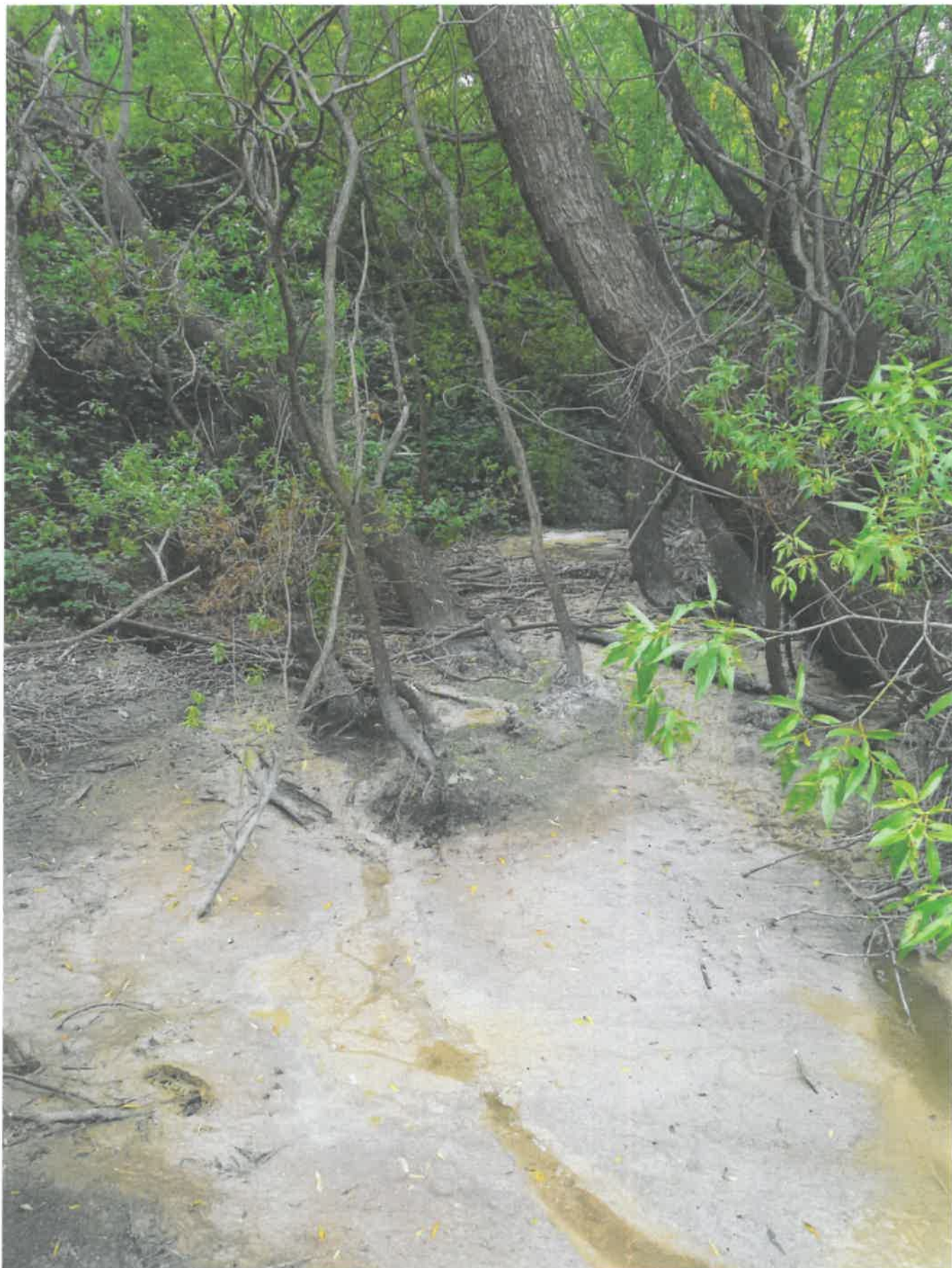
View from upstream side of sewage discharge looking back towards stormwater pipe (centre left of photograph) that was discharging sewage. Note sludge in foreground.
