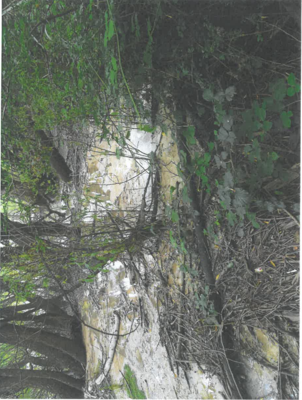
View from beside stormwater pipe outlet on right, looking towards the Kawarau River, showing the sewage discharge.
