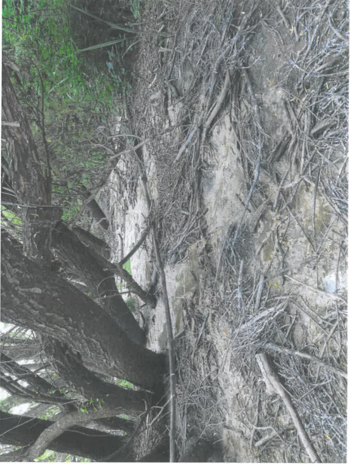
View from downstream looking back at stormwater pipe outlet (top right behind the bushes).
