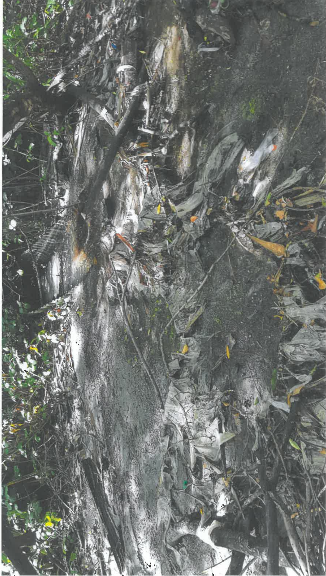
View showing clear water leaving the stormwater pipe outlet, but toilet paper and sewage was caught in sticks, pools of sewage sludge everywhere.
