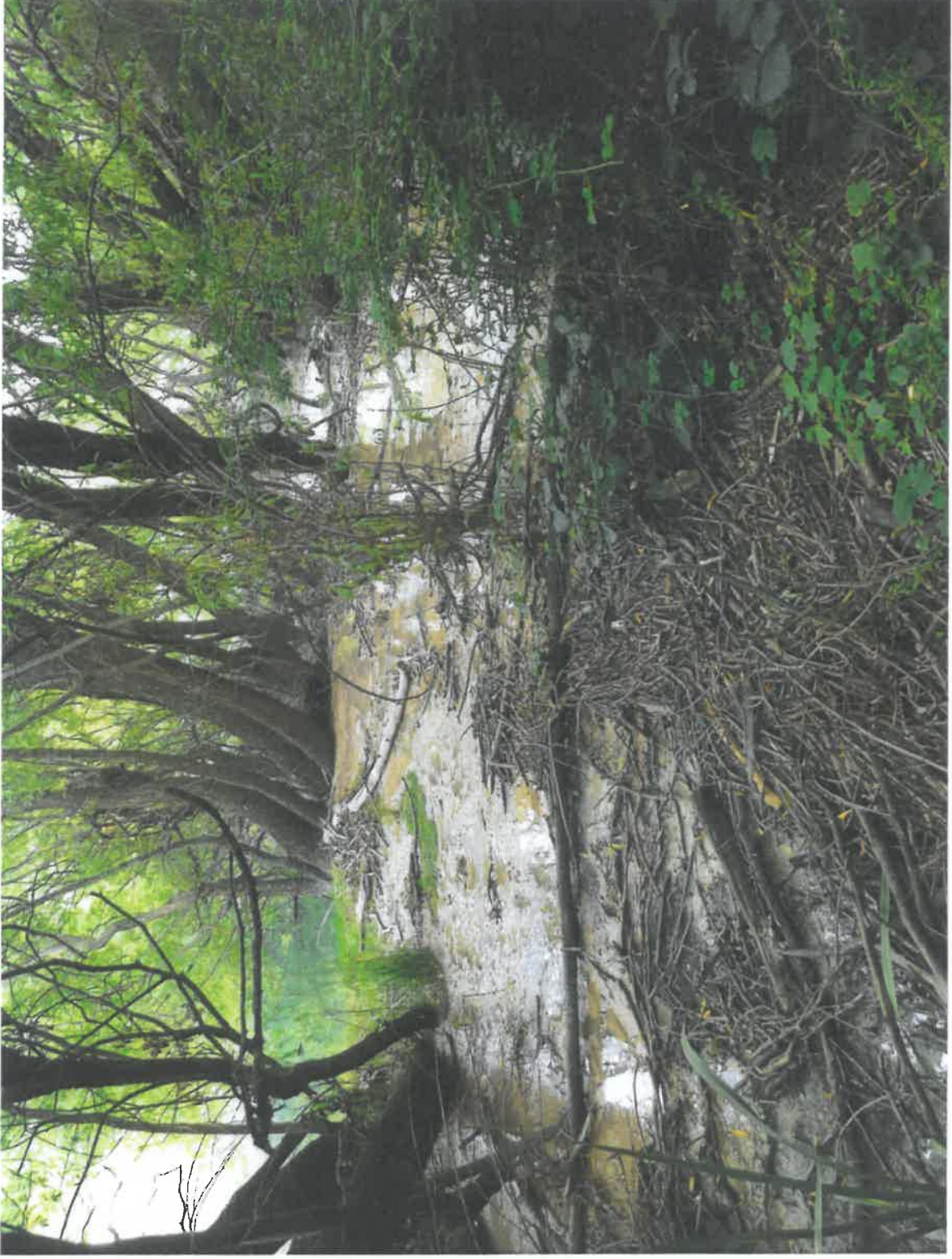
View of sewage flowing from stormwater pipe outlet on right looking towards the river, showing sewage flow path. Similar to previous photograph.
