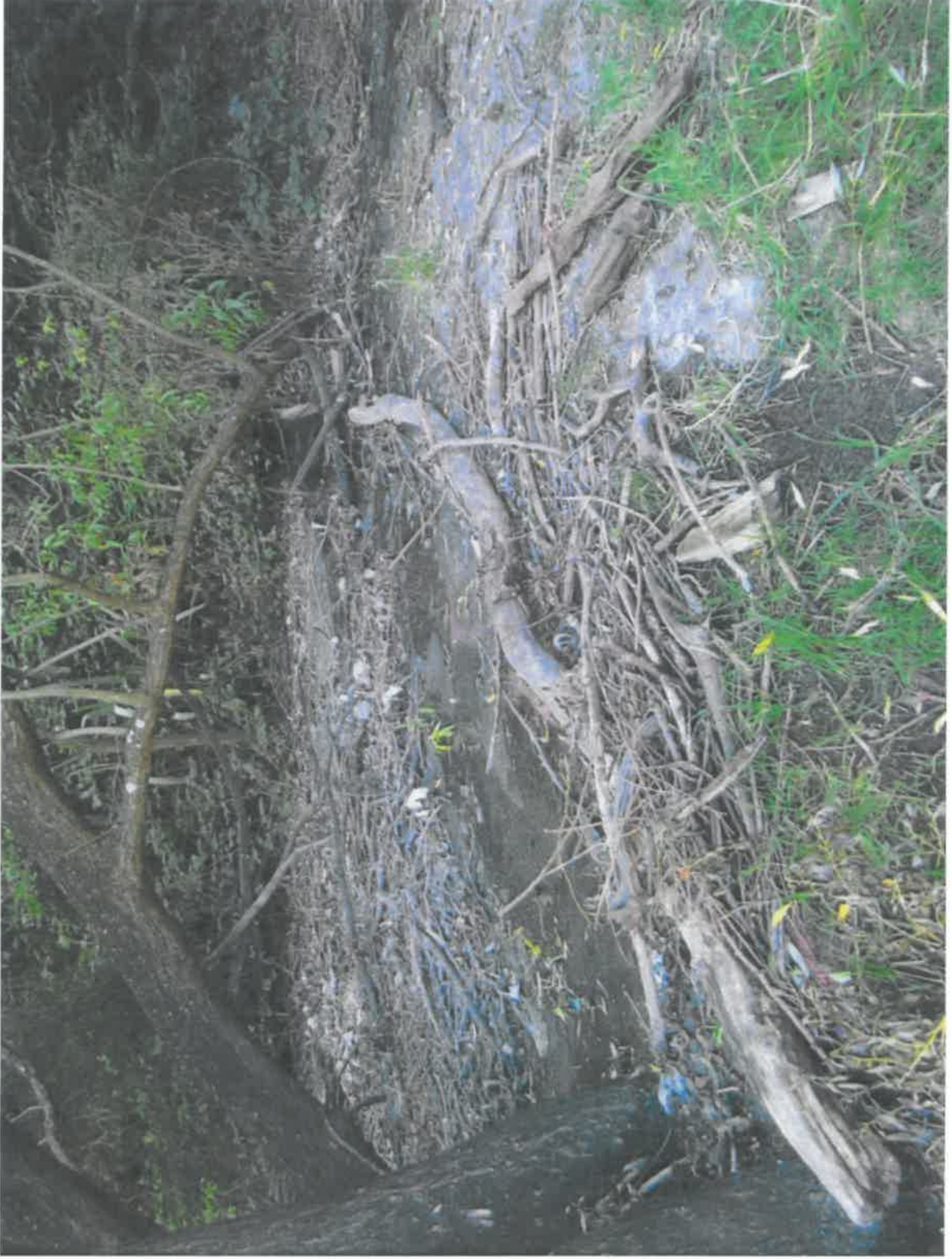
View looking back towards the stormwater pipe outlet where the sewage discharge occurred. Shows area of ponding and flow paths left and right from outlet.
