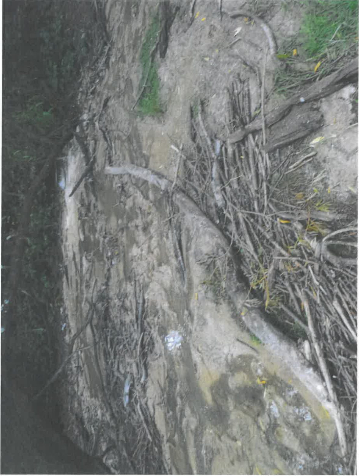
View from green mound looking back towards the stormwater pipe outlet, showing sewage sludge.
