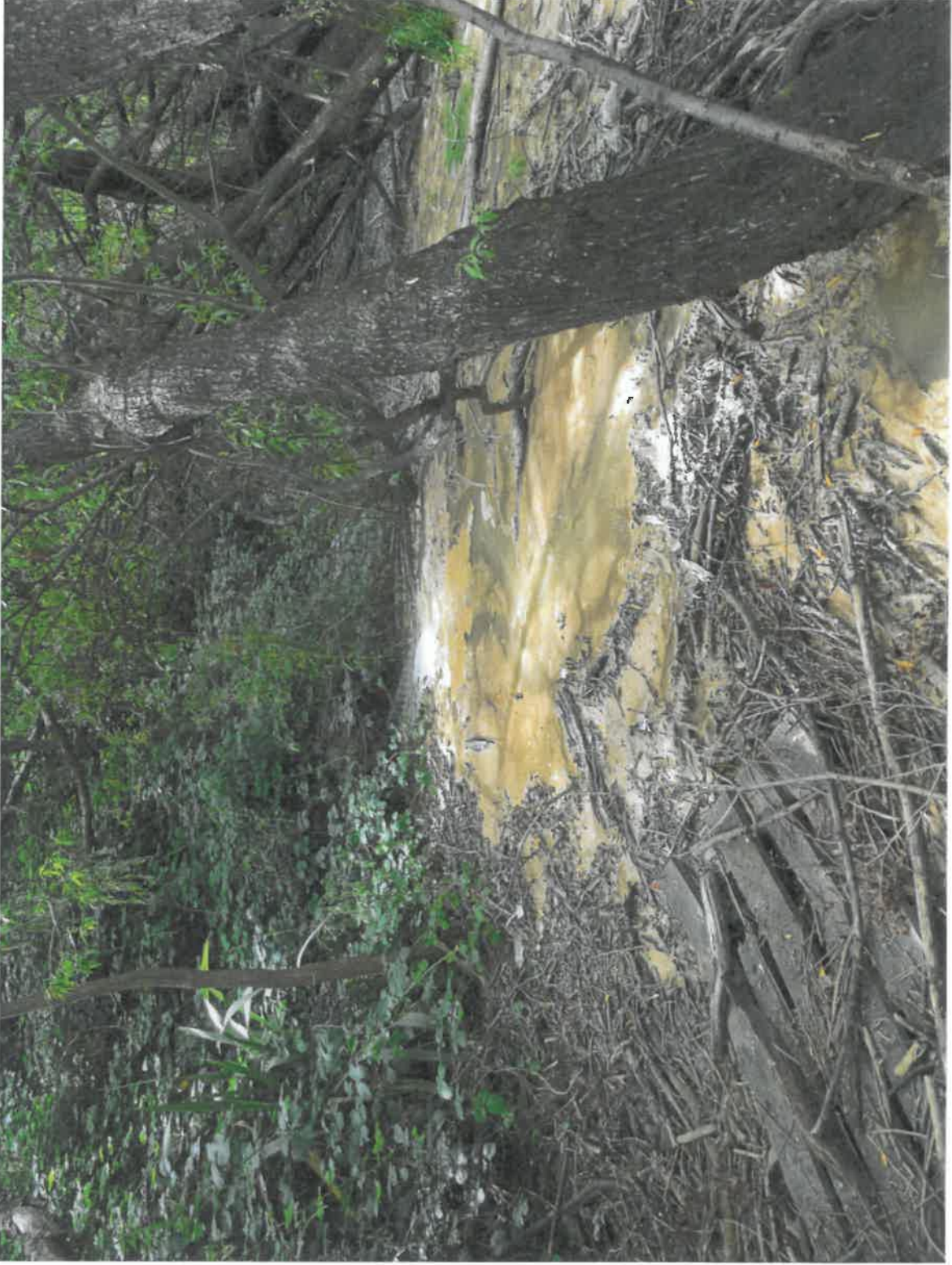
View from upstream side of the sewage flow to river, looking back towards the stormwater pipe outlet at middle centre.
