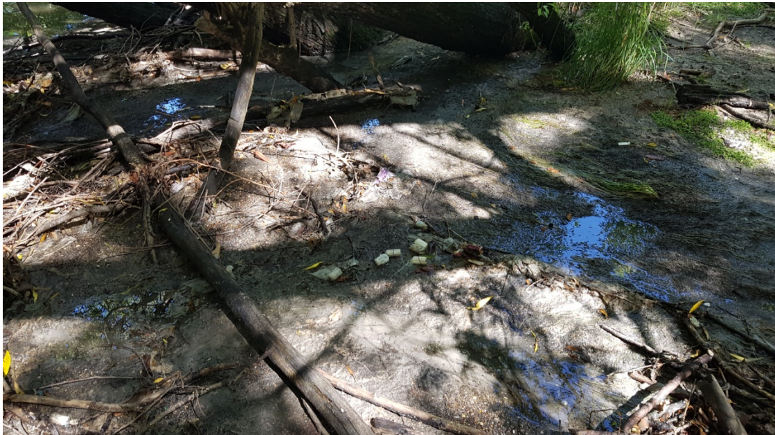
Photograph 1 Discharge to Kawarau River 1 showing overflow containing female sanitary products
