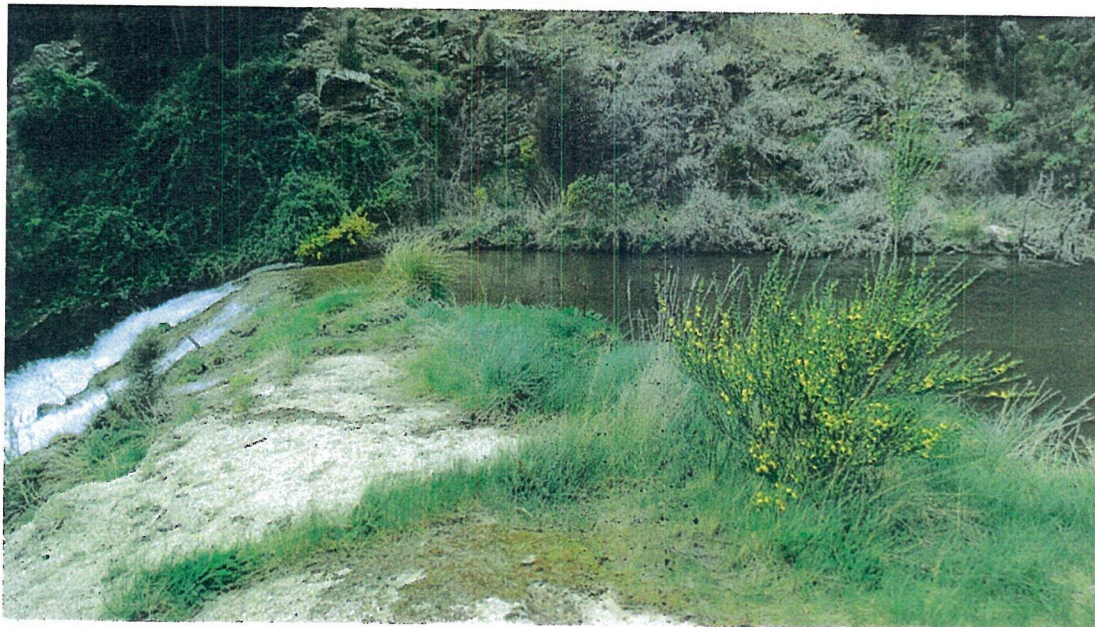
Photo looking along weir crest from true left bank to right bank of intake weir
