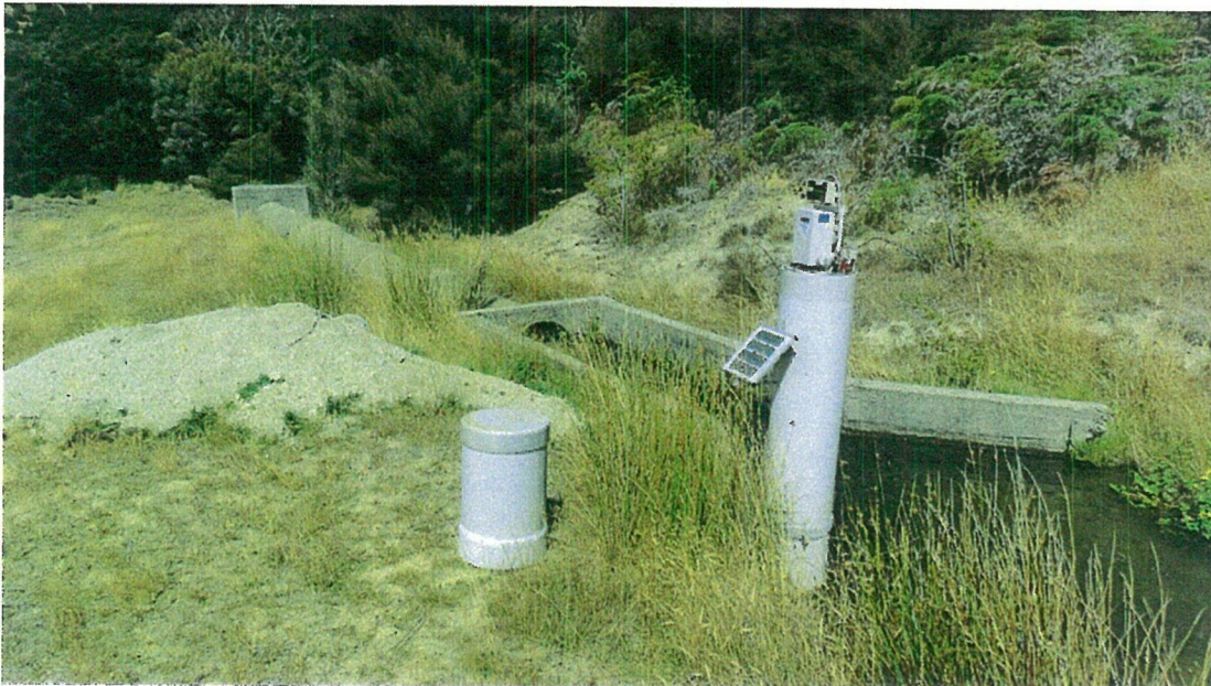
View from north looking SE at outlet end of 490m concrete supply pipeline from Luggate Creek weir. Flow splits downstream of this point. Water measuring equipment in foreground. Photo 28 October 2014
