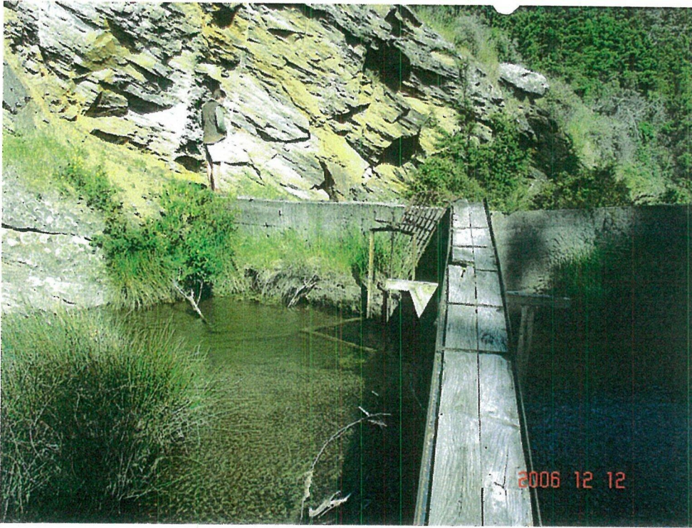
Intake control gate at Luggate Creek weir left bank and sump inlet to 685mm diameter concrete pipe to water measuring site, some 490m downstream. Looking NW along walkway to control gate for through-weir discharge pipe. Photo 12 Dec 2006
