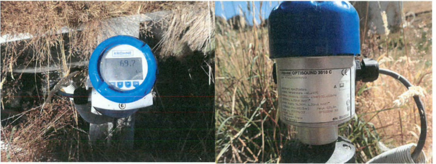
Water meter for both takes E1303023 N5037743.
