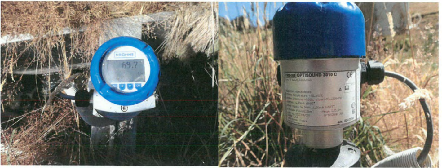
Water meter for both takes E1303023 N5037743.
