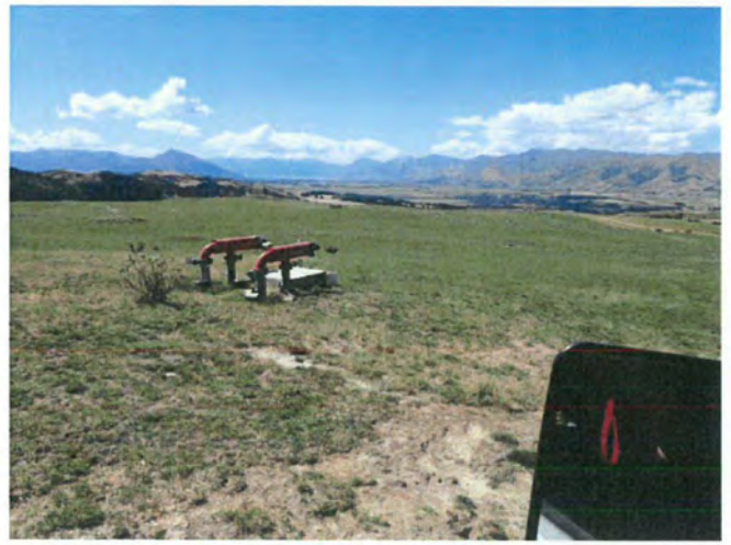
Filters before water goes through irrigation system.
