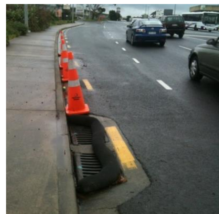
Figure 98: Installation of a silt sock to provide some protection to the catchpit
