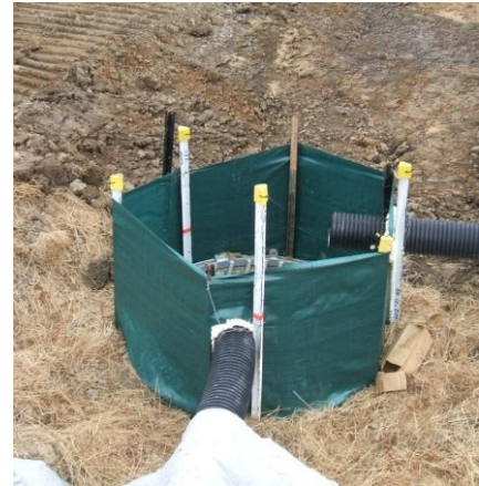
Figure 97: Good use of a silt fence installed to protect a new stormwater catchpit where impounded water will not create a flooding hazard
