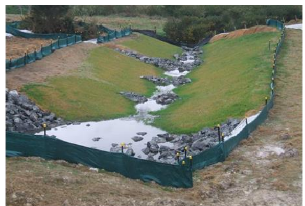
Figure 25: Check dams installed in series to act as a permanent water velocity control measure
