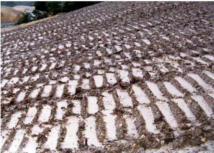
Figure 39: Surface roughening of a slope. Note the hollows acting as "micro" sediment traps
