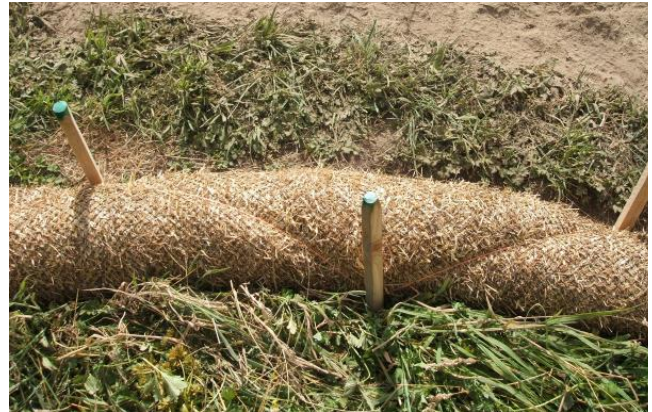
Figure 93: Straw sock secured in place using stakes and bale twine; note the stakes are placed every 600 mm
