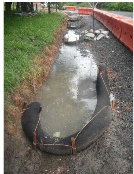
Figure 26: Silt socks can be used as a check structure on a low gradient channel
