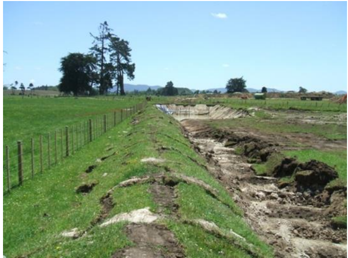
Figure 15: Turfing scraped from within the site to stabilise the perimeter bund. The perimeter bund provides both clean and dirty water control
