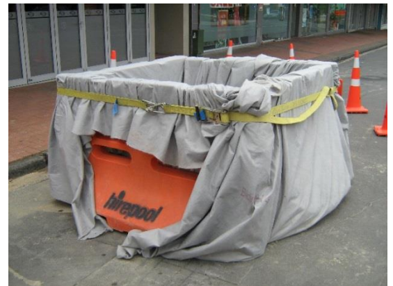
Figure 106: Example of a mobile 'turkey nest' used for dewatering
