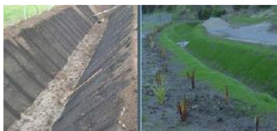
Figure 63: Bonded synthetic fibre mat used as erosion protection and medium for revegetation
