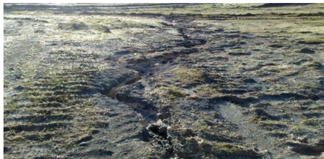
Figure 46: Loss of topsoil and grass seed after heavy rain event. Will require stabilisation and reapplication
