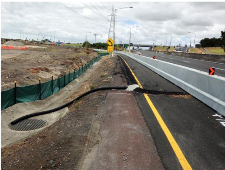
Figure 17: Hotmix bund diverting the motorway runoff to the catchpit
