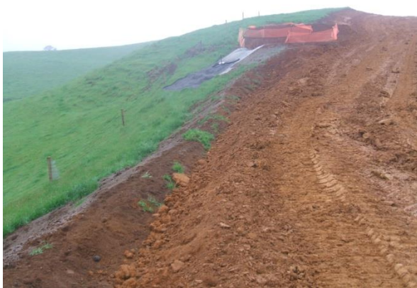
Figure 123: Decanting earth bund and diversion bund installed during a farm track construction
