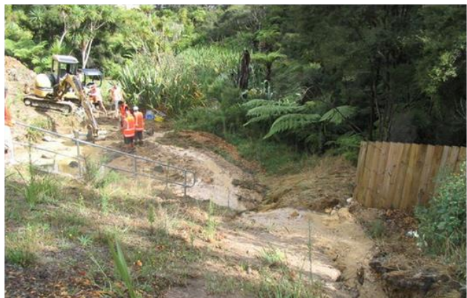
Figure 12: Sediment discharge as a result of not protecting the watercourse
