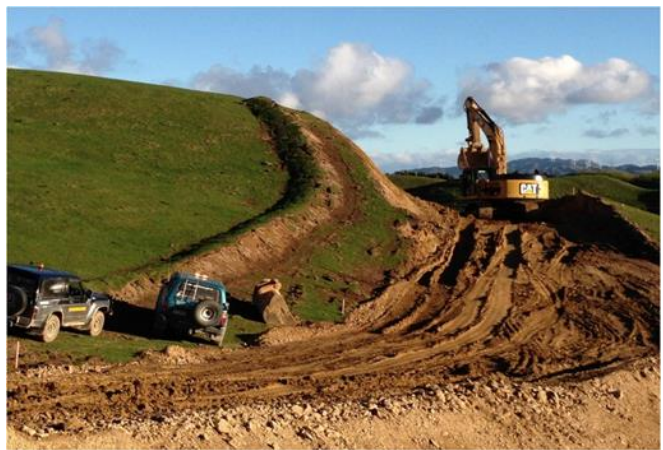
Figure 14: Clean water diversion used to isolate upper clean water flows from the works area
