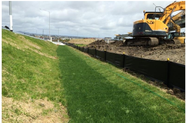
Figure 52: Turf used to provide instant stabilisation of the swale allowing for early commissioning of the device
