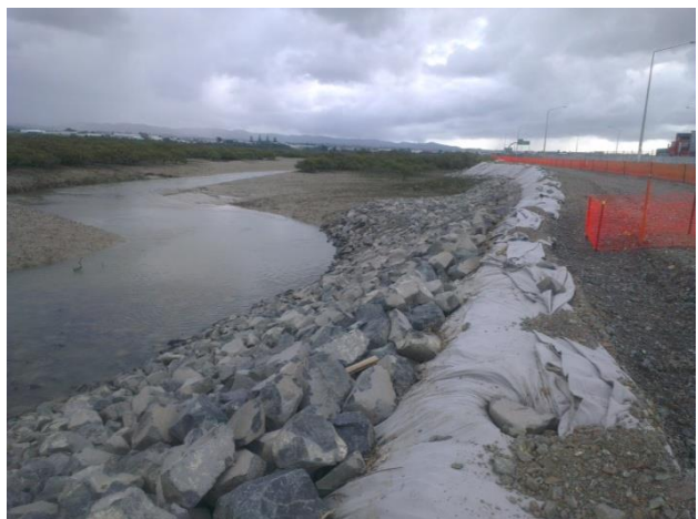
Figure 130: Examples of geotextile filter layer beneath a rock revetment and use of rip rap
