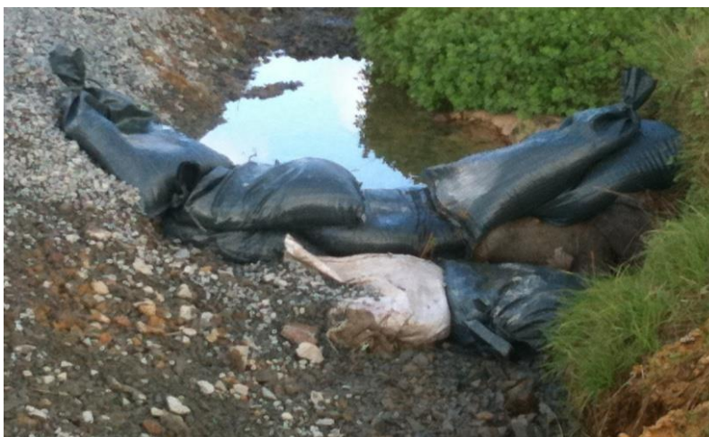
Figure 27: Check dams installed with a spillway to direct flows over the centre of the structure. Sand bags placed directly below spillway provide a protective apron below the dam
