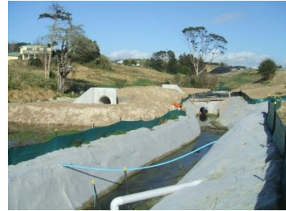
Figure 112: Stabilised clean water diversion and temporary culvert to divert streamflows while a new culvert is being constructed
