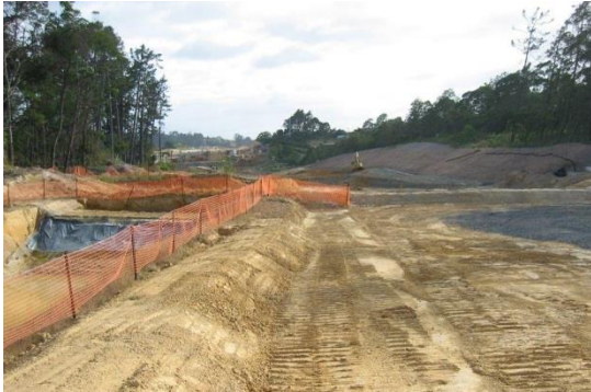
Figure 19: Dirty water diversion bund directing site water to a sediment retention pond
