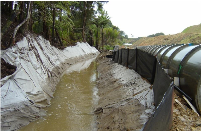
Figure 111: Temporary stream diversion to allow for the installation of a new culvert
