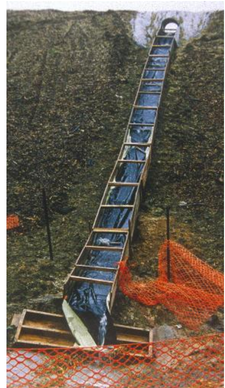
Figure 31: Wooden flume lined with impervious material
