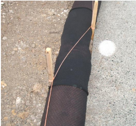
Figure 92: Silt sock joined using a sleeve and pegged and secured using bailing twine with 1 m overlapping joint
