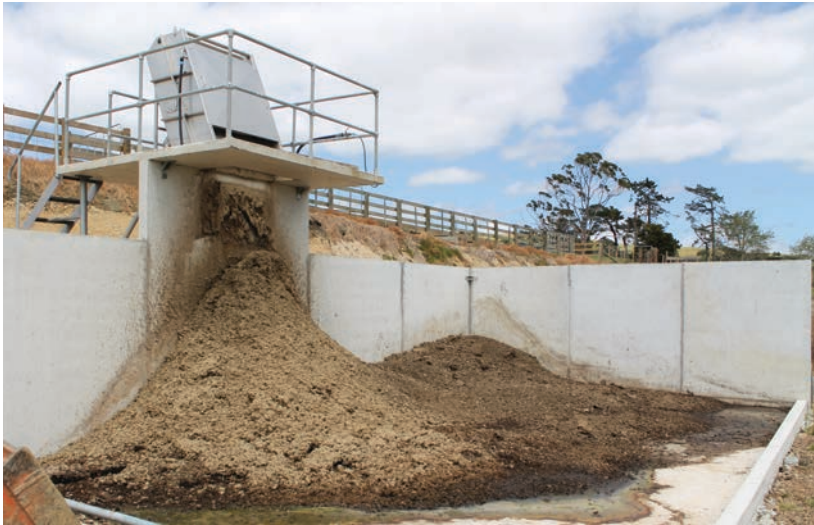
Typical static screen and bunker installation
