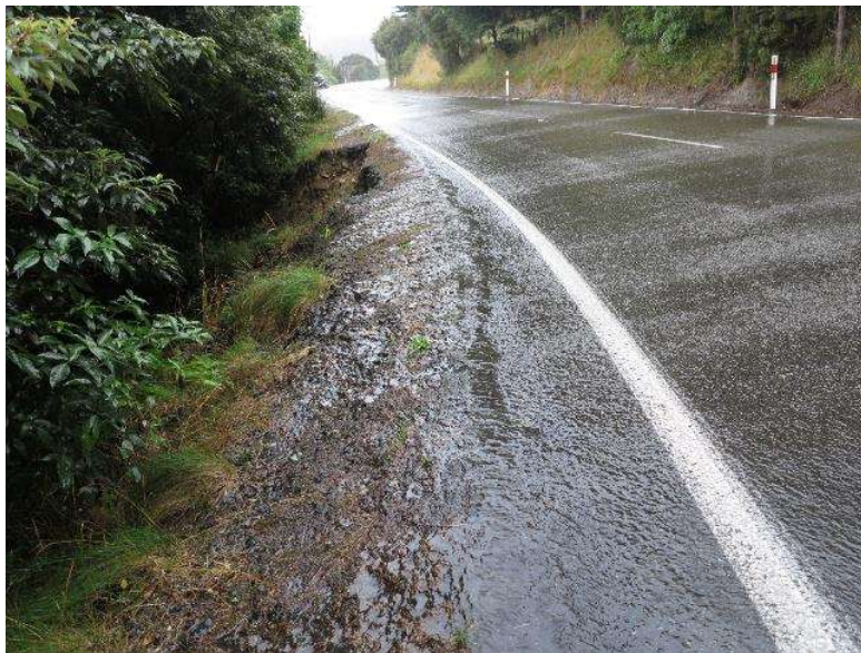
Figure 3-10: Slip beside Blueskin Road (photo February 2020)
