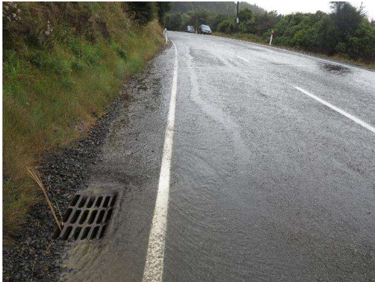
Figure 3-9: Inadequate drainage along Blueskin Road
