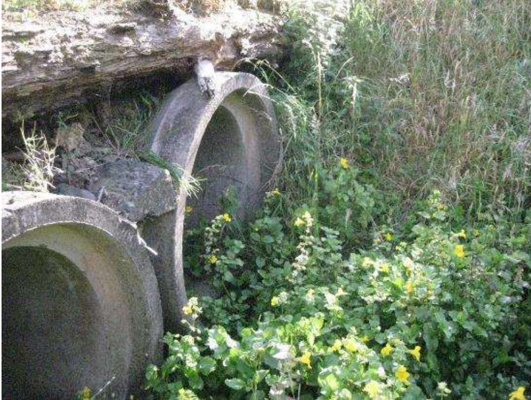
Figure 3-12: Rotting headwall pole, collapsing dry stone wall and plant obstruction
