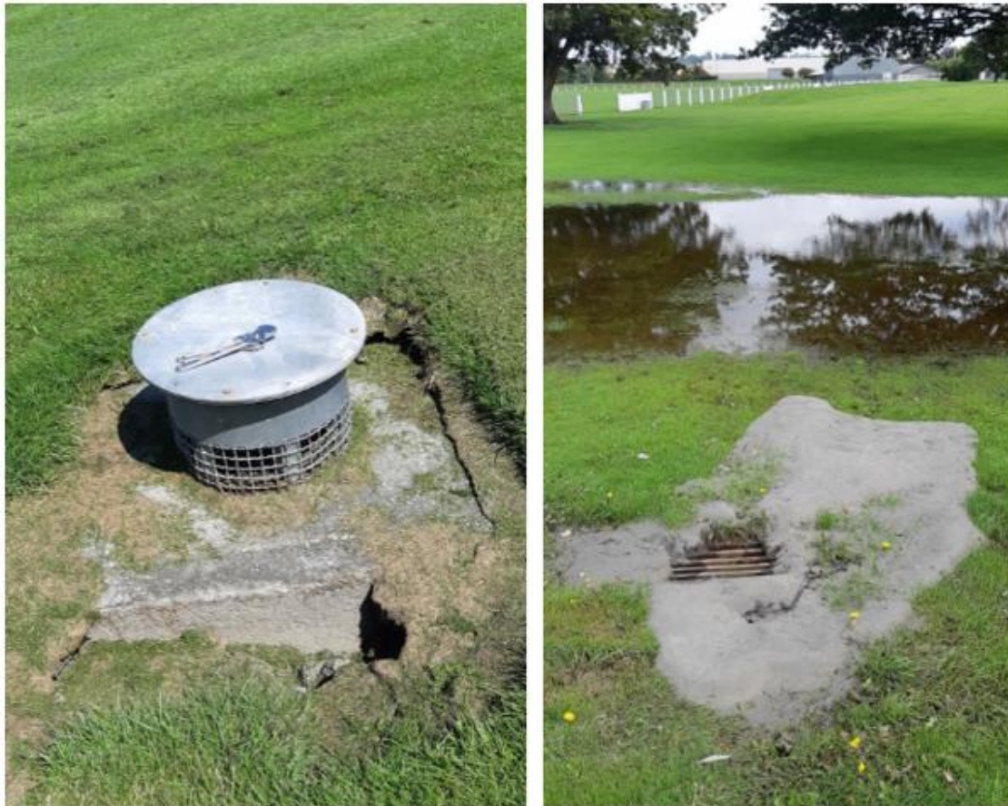
Figure 7. Balclutha stopbank pressure relief wells; near swimming pool (left) and near recreation hall (right)
