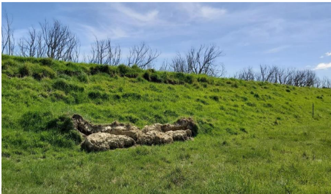
Figure 6. Slumping and toe bulging on landside toe of Waitepeka floodbank.
