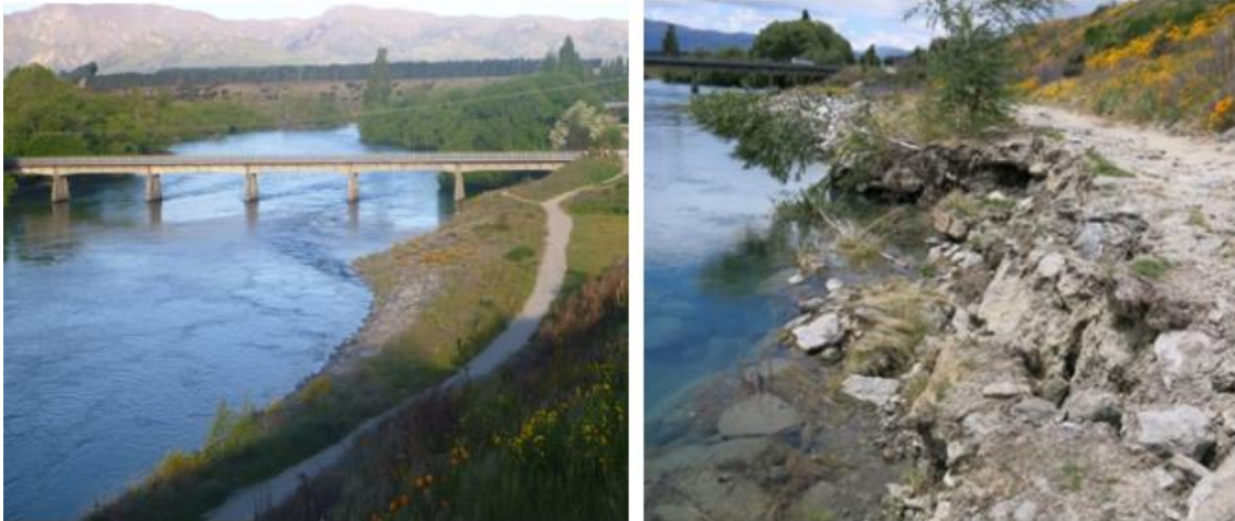
Figure 8. Albert Town Rock Buttress providing protection upstream of SH6 (left) and damage to rock and slumping (right).
