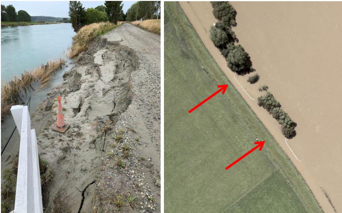
Figure 3. Slip damage on Riverbank Rd (left) and inundation of Riverbank Rd at the height of the 5 February 2020 Flood.
