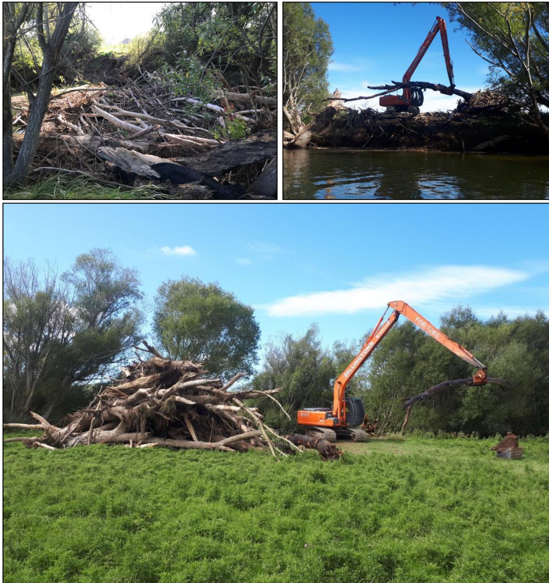
Figure 10. Debris before, during and after removal from Pomahaka River, near Winslade Road, Kelso.
