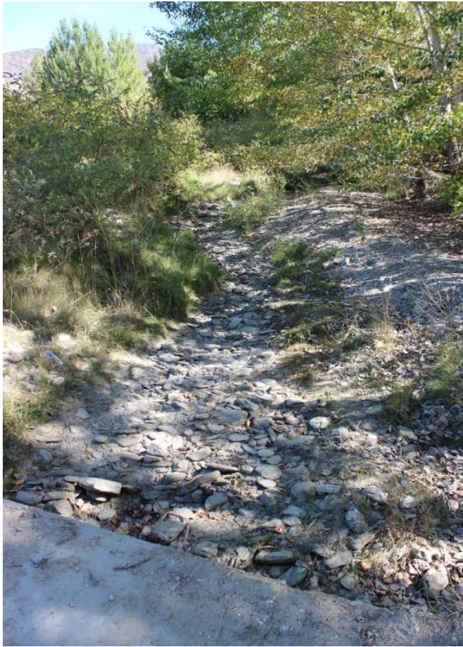
Figure 8: Long Gully at the location of Photo 7 in the map above (Black Quail Culvert) – looking upstream.
