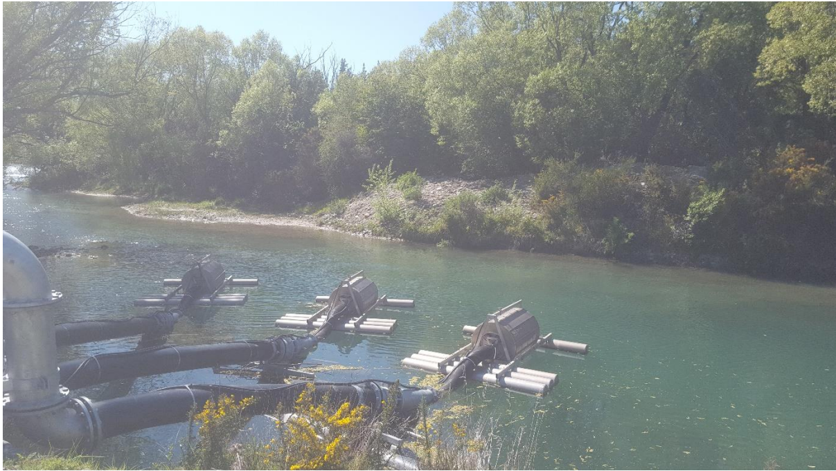
Figure 8: Three pumps installed in the small channel of the Clutha River that pump water to the Peninsula pivots and the tank farm (October 2018).
