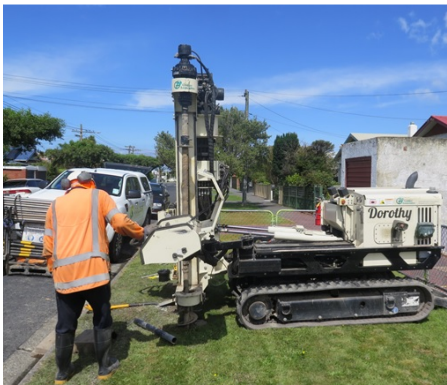
Figure 1. Cone Penetrometer Testing (CPT) rig taking pressure readings from the soil beneath South Dunedin in 2019.
