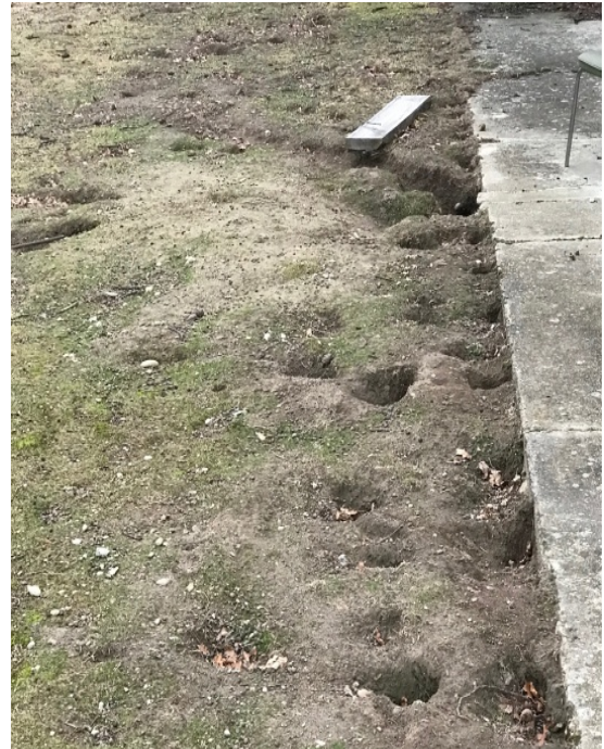
Rabbits had been undermining hospital buildings, fences and lamp posts.
