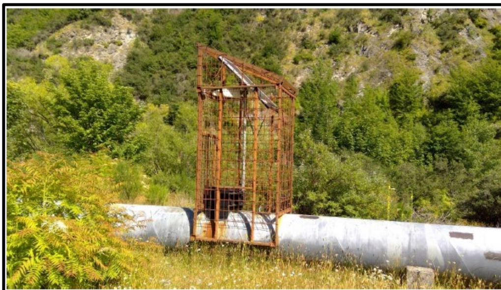
Image 4: Water meter on delivery pipeline (Source: Application)
