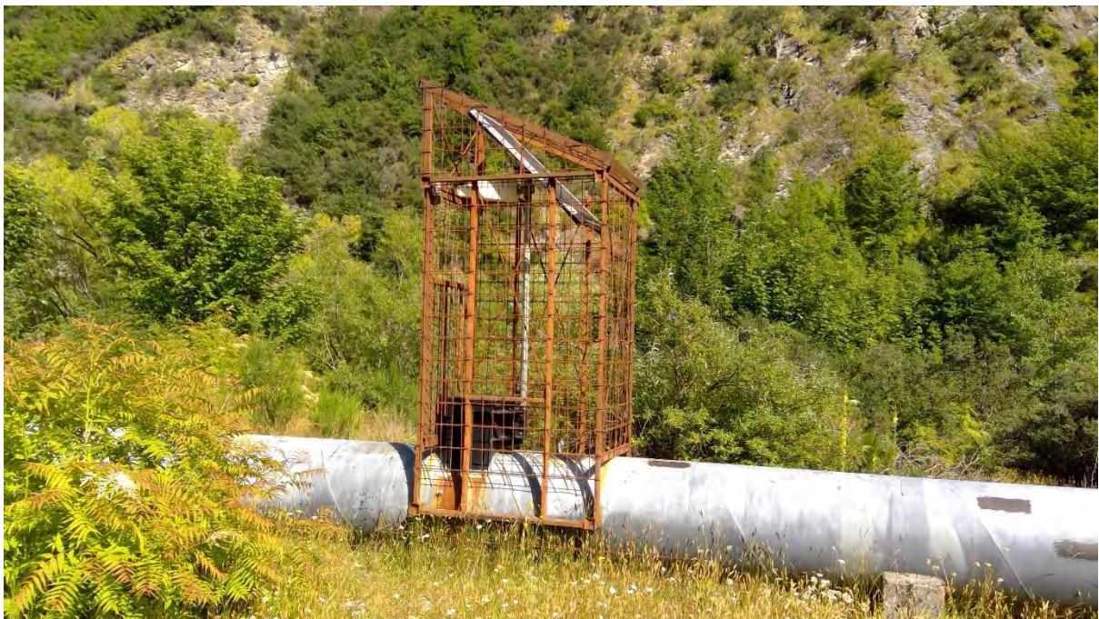
Plate 12: Water Meter, delivery pipeline
