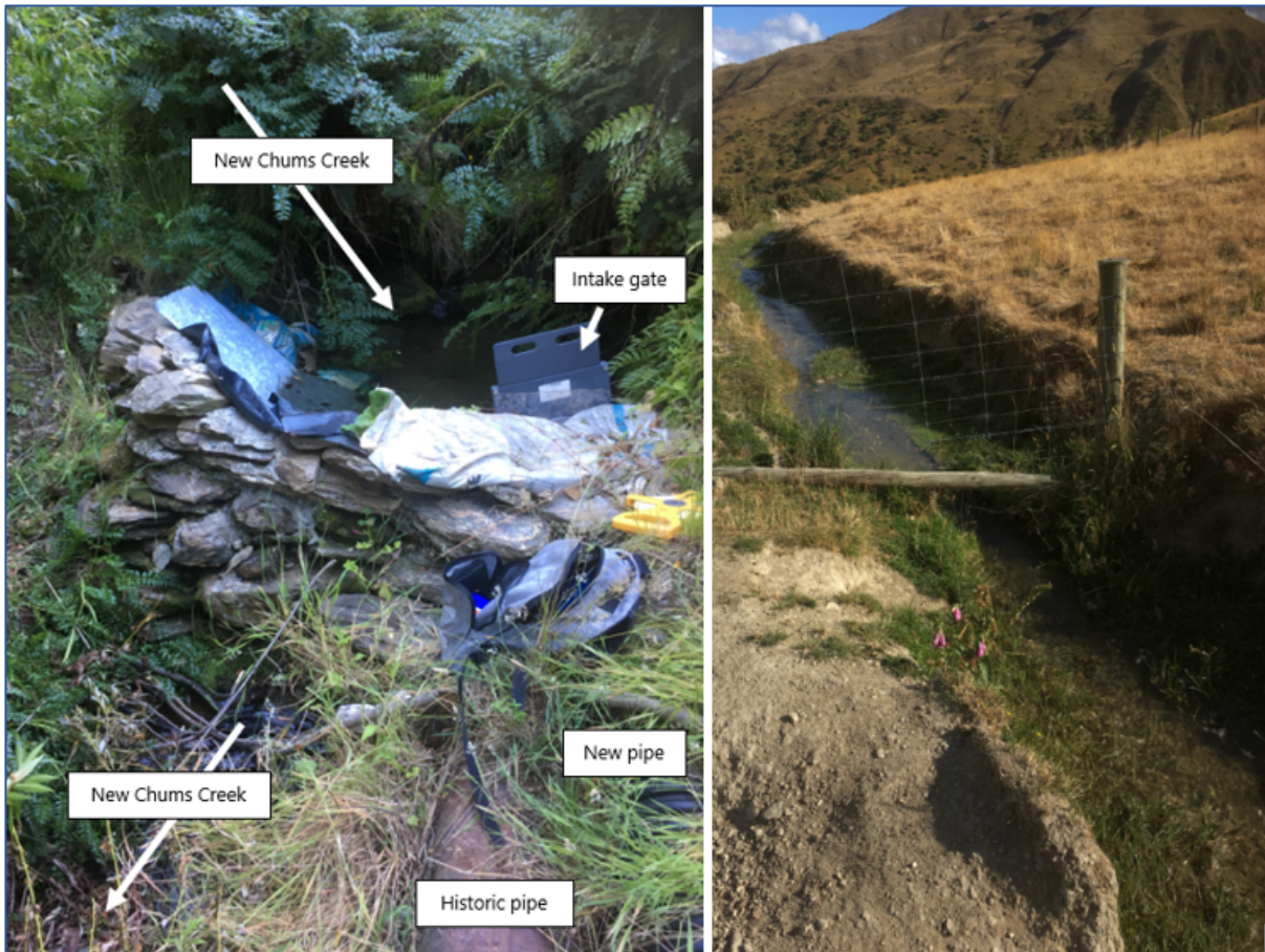
Figure 4: Intake structure on New Chums Creek (left) and New Chums Race (right)
