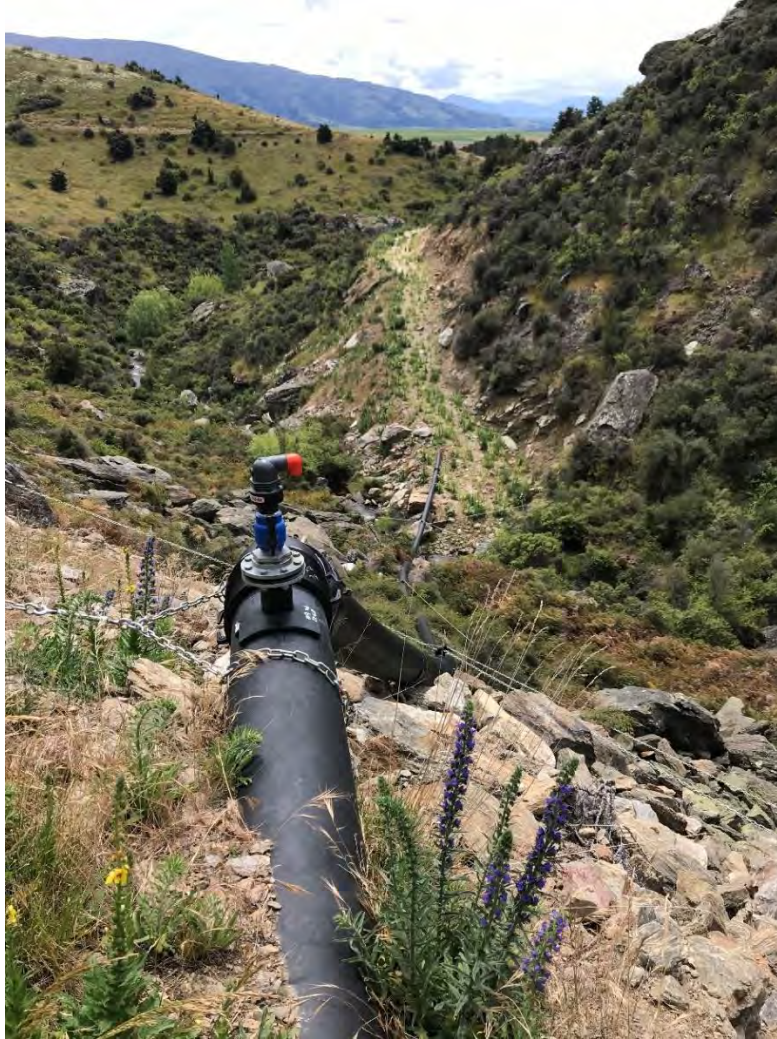
Figure 4: Pipeline carrying water abstracted from Bendigo Creek. The pipeline generally follows the old water race route.
