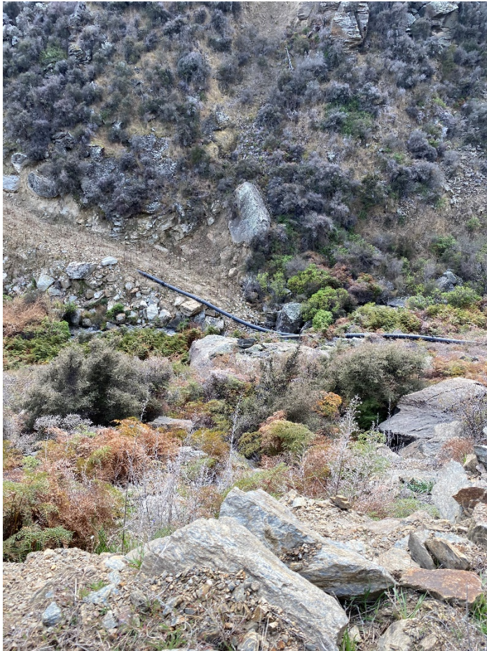
Figure 5: Pipeline conveying water from the point of take across Bendigo Creek towards the ponds/junction box.
