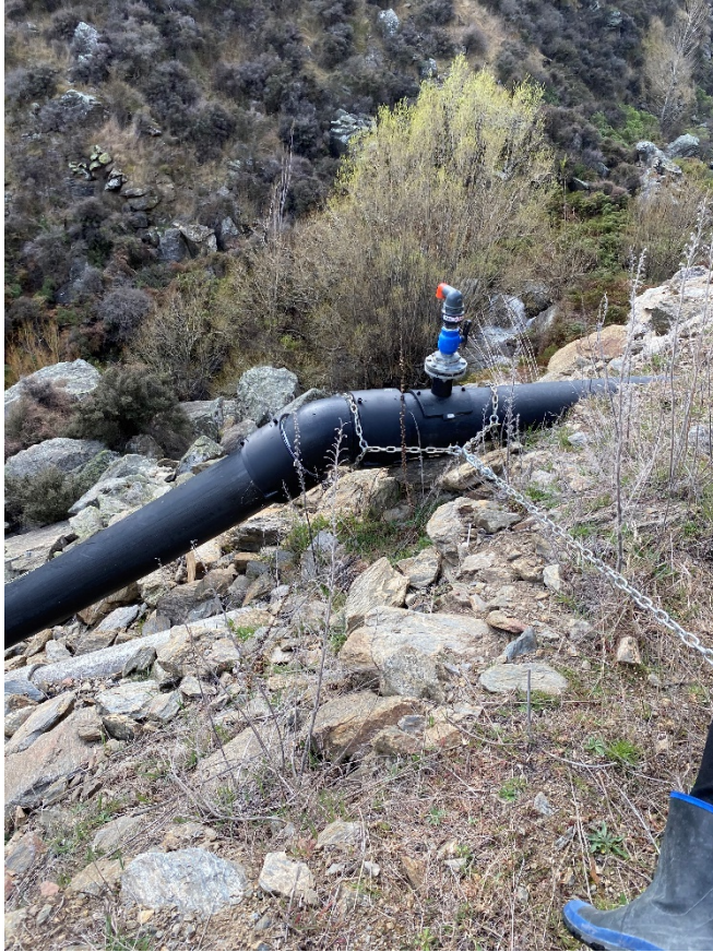
Figure 4: Intake pipe with control valve.
