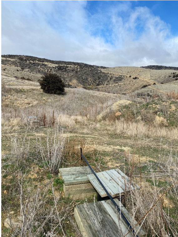
Figure 6: Second valve, junction and meter.
