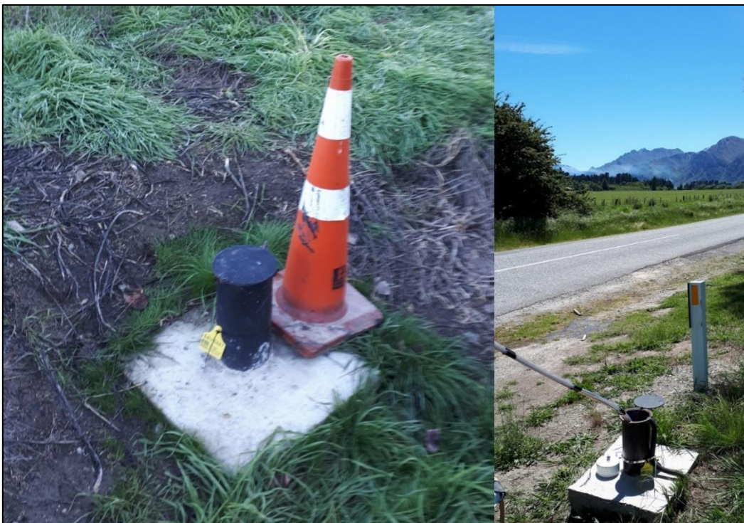
Figure 2: Examples of suitable, secure, purpose-drilled monitoring bores. Note the sealed concrete pad surrounding the bore head, raised casing above ground level, and the lockable cap.
