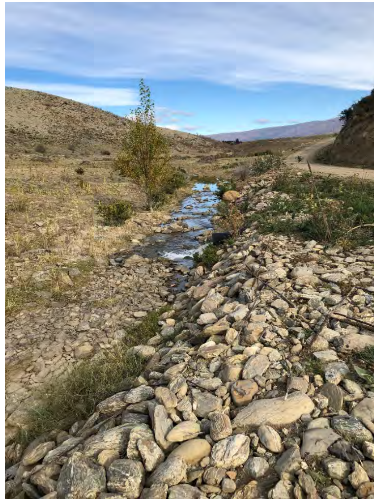
Image 2: Looking west showing the culvert (midway point of image) that runs through the formed road providing water back into Bendigo Creek.
