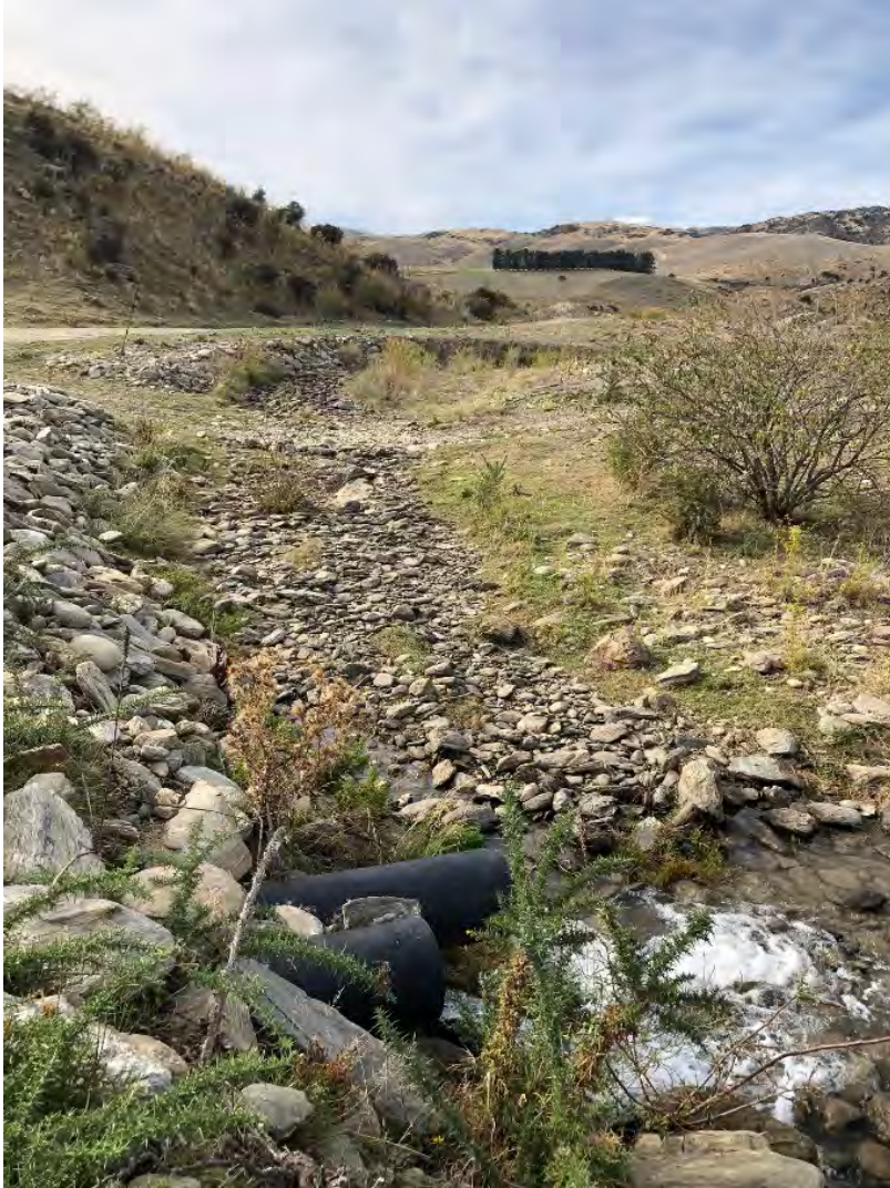
Image 3: Looking south-east identifying Bendigo Creek running dry with culvert Supplying stock water back to Bendigo Creek.
