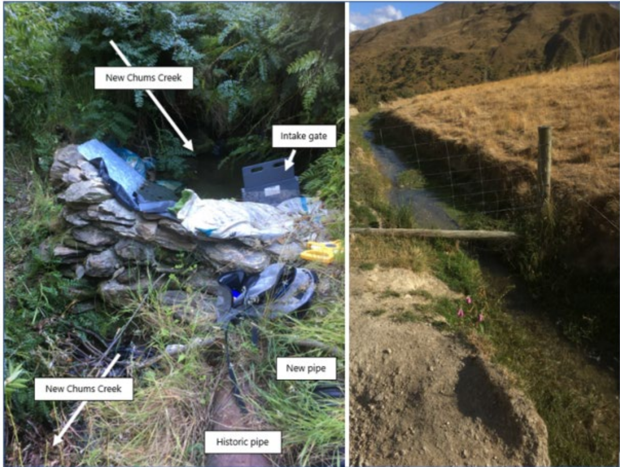
Figure 6: New Chums intake showing the intake gate, new pipe and historic pipe. Source: Application.
