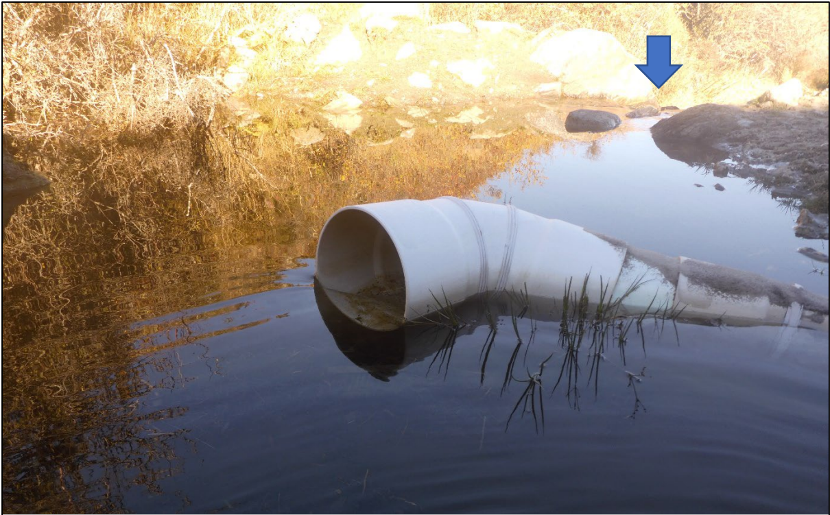
Figure 3: Pipe intake at upper Royal Burn North Branch water take. Intake pipe diameter is 330 mm. Outflow of ponding area is shown by blue arrow. Photo taken by Bryony Miller during site visit 13/05/2021.
