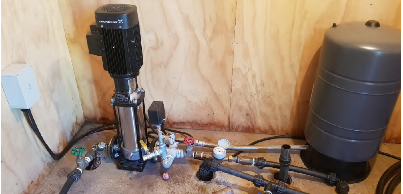
Figure 4: pump and water meter
