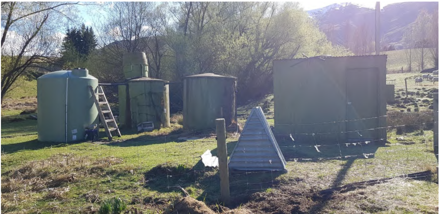
Figure 3: pump shed and 3 settling tanks
