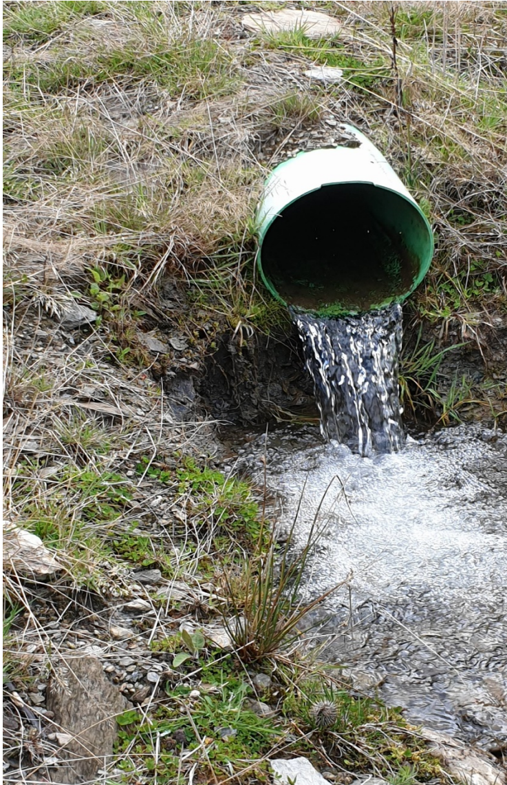
Photograph 4: View looking at discharge from New Chums Creek at point downstream from the Parshall Flume shown in Figure 2. Pipe is 280 mm in diameter.
