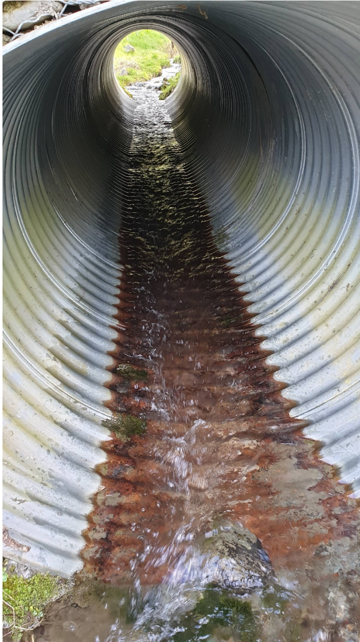
Photograph 8: View of downstream exit of culvert under Glencoe Road for the Royal Burn South Branch. Culvert is 545 mm in diameter. As can be seen from the heavy iron staining and the moss on the inside of the culvert, the flow is seldom much greater than this. This is Location 1 on Figure 3.
