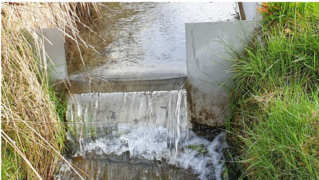
Photograph 11: View of rectangular weir. Weir crest is 500 mm wide.
