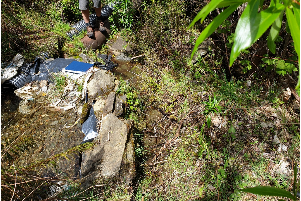
Photograph 1: View of intake dam at New Chums Creek. Black corrugated pipeline is new and the old, abandoned iron pipeline is supporting the person. As can be seen the downstream face of the “dam” is lined with plastic sheeting to prevent as much water as possible to be directed down the pipeline. New Chums Creek bed is evident on the right-hand side of photograph but has minimal flow down it at the time the photograph was take.
