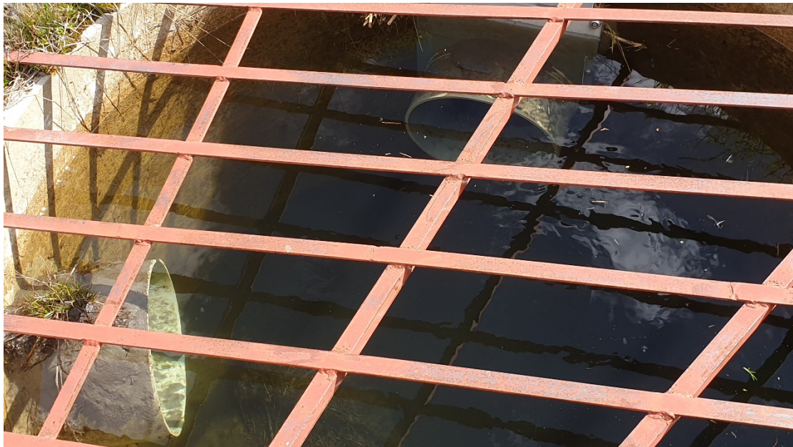
Photograph 7: View looking at collection chamber with inlet pipe on the left-hand side and the outlet pipe at the top. Flow is controlled using a movable plate which is inset in the outlet pipe. No flow measurement is done at this point, so any adjustments require at least two people to do accurately. This chamber is only slightly above the water level when the photographs were taken so the flow cannot be much more than this at any time during the year.
