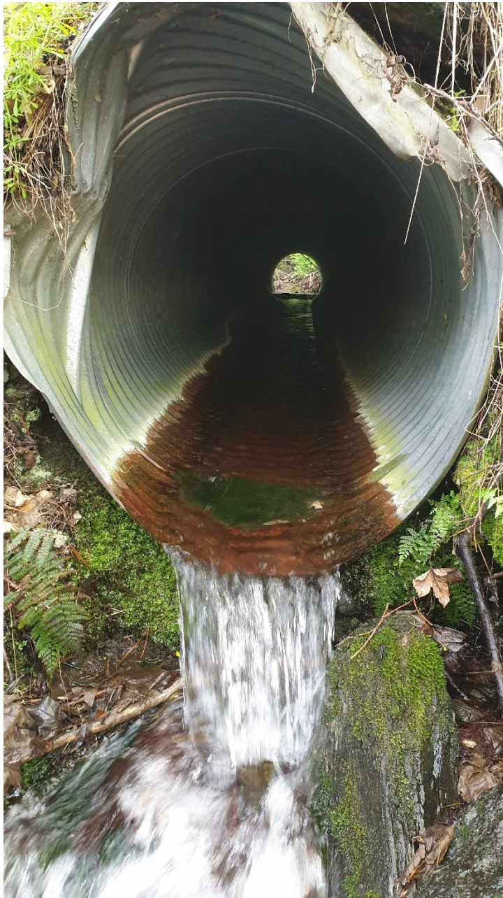
Photograph 9: View of downstream exit of second culvert under Glencoe Road carrying flow from Royal Burn North Branch. Location 2 on Figure 3. Culvert is 545 mm in diameter. As can be seen by the iron staining and moss growth on the sides of the culvert, the flow is seldom greater than that shown.
