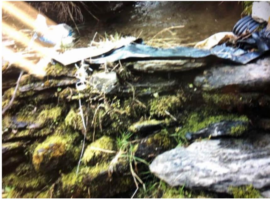
New Chums Creek Outtake Seepage (less than 5% through dam wall)
